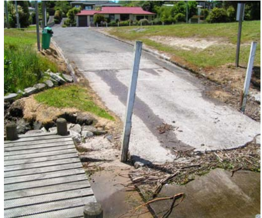
Figure 18.1. Seep emerging from boat ramp just west of Hamurana. Water is seeping out of cracks (centre) and both sides of ramp. Trough is to the east of the ramp.
