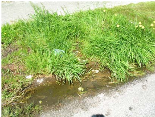
Figure 1.1. Seep in gutter outside 60 Pohutukawa Drive, Rotorua.
