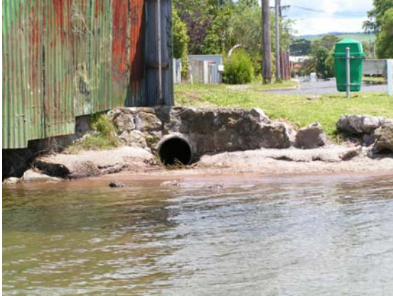
Figure 67.1. Roadside runoff drains through pipes into lake.
