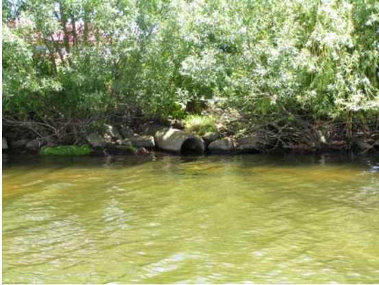
Figure 62.1. Drain at south end of Lake Rotorua.
