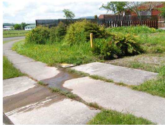
Figure 1.2. Seep on driveway of 60 Pohutukawa Drive, Rotorua.
