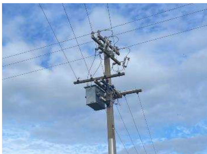
Figure 6 - Example of the small-scale transformers observed throughout the region
