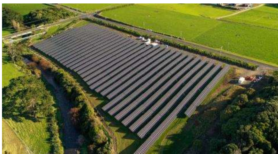
Figure 2 - The Kapuni Solar Power Plant, a utility scale ground mount array installed by Sunergise, utilising a fixed tilt configuration.
