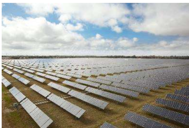
Figure 3 - A ground mounted array in a single axis tracking configuration
