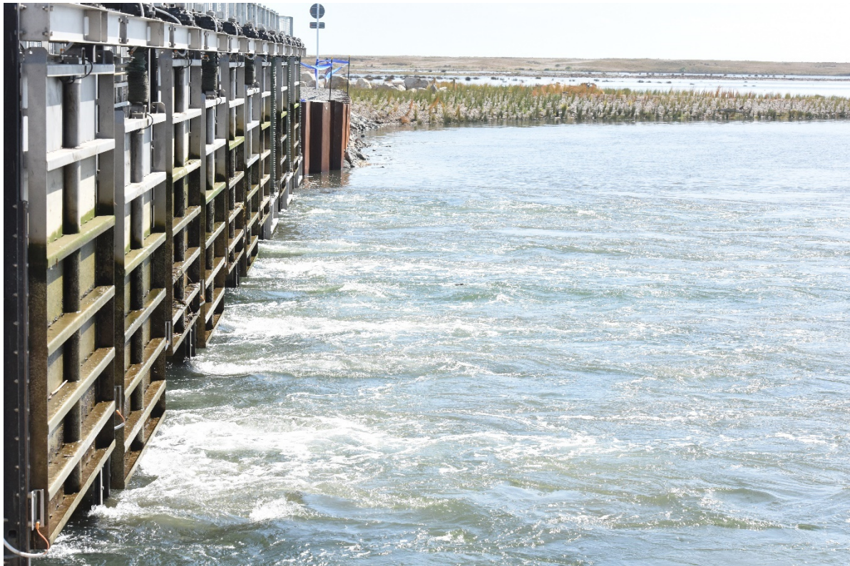
Figure 3: Control gates open into Ford's Cut and estuary (© Bay of Plenty Regional Council – Reprinted with permission)
