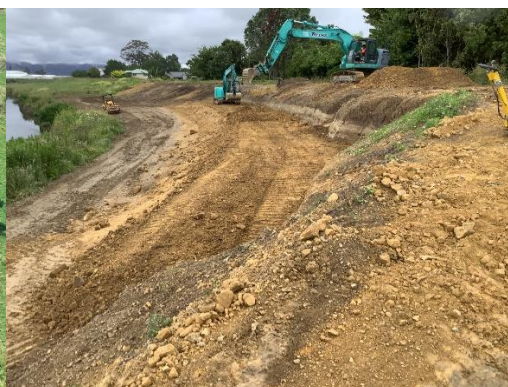
College Rd identified asset defect repair
