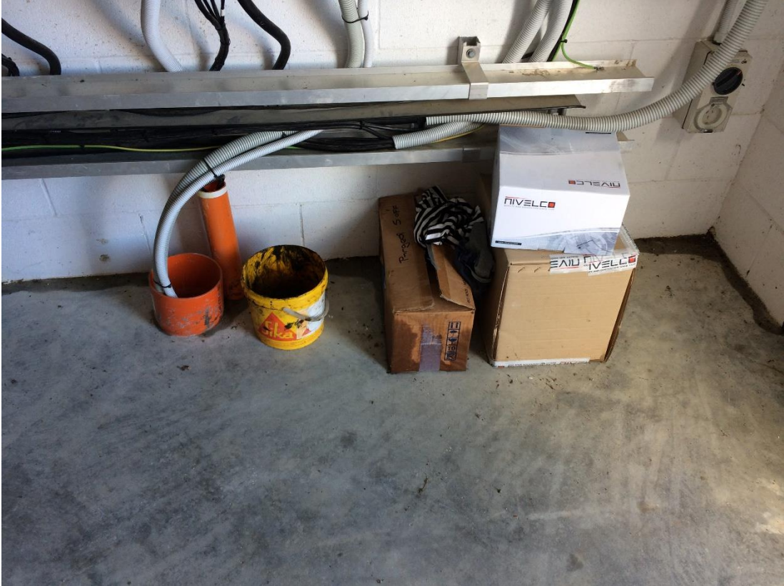
Photo 13: Control building moisture
