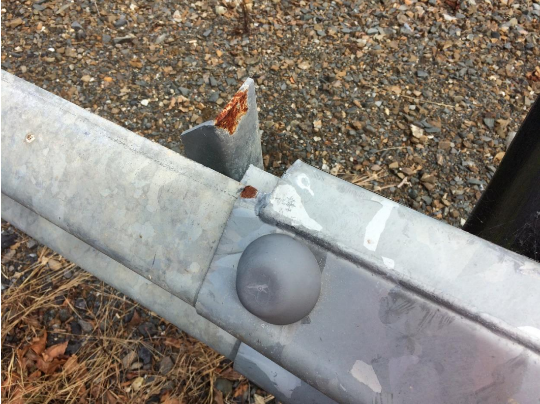
Photo 27: Guard rail post corrosion
