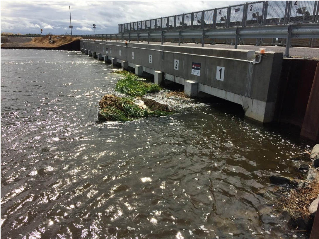
Photo 14: Weed raft across culverts
