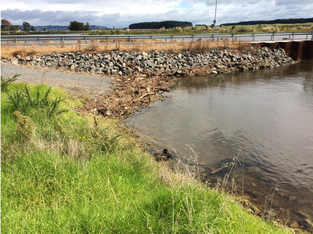
Photo 15: Debris downstream of culverts
