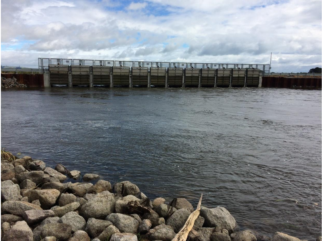
Photo 16: Debris impeding culvert flow
