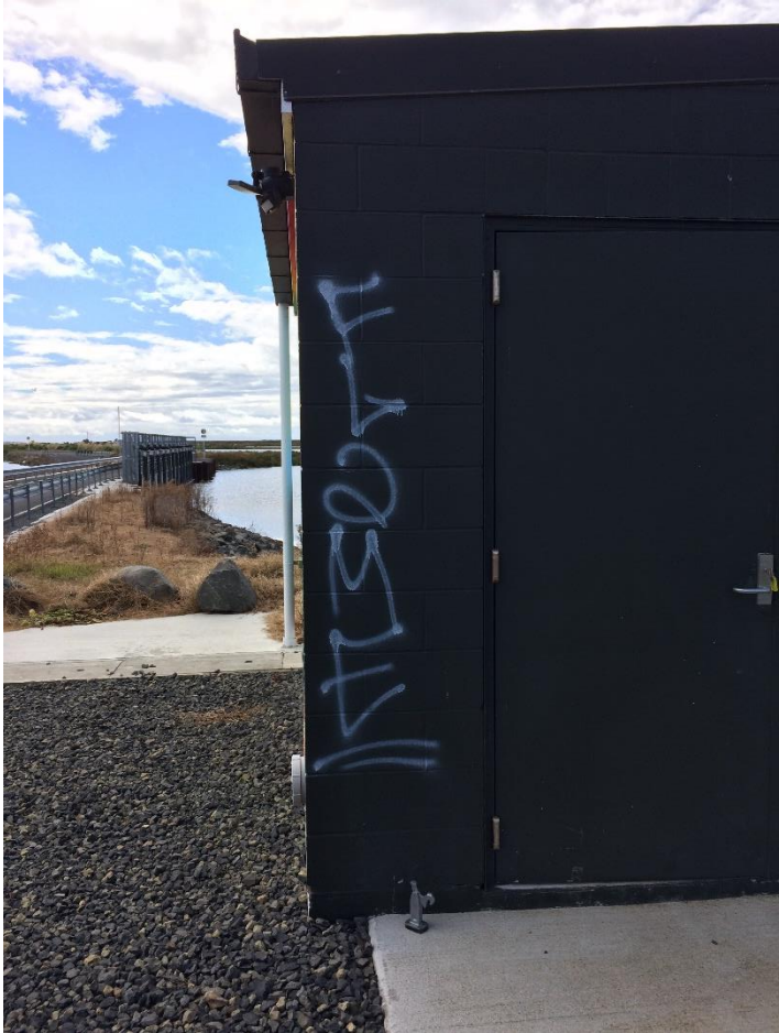
Photo 12: Control building graffiti
