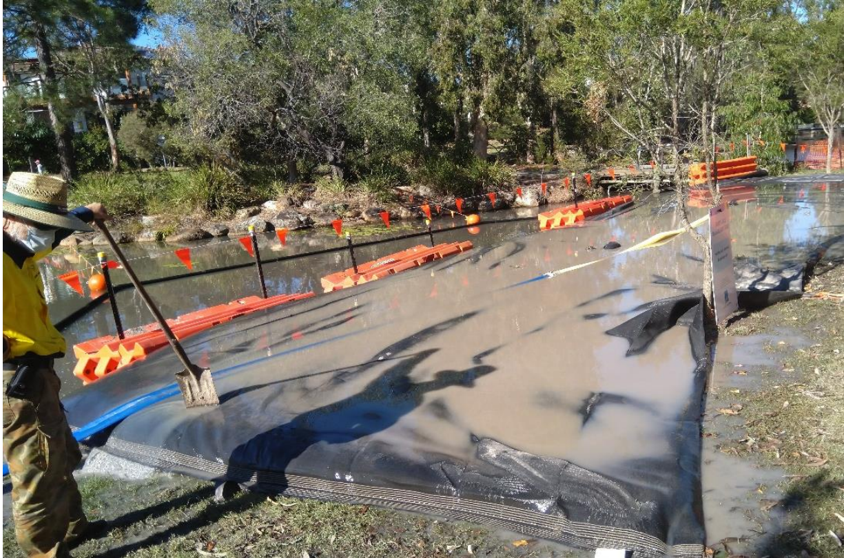
Figure 9 A sediment removal operation in Forest Lake, Brisbane, Australia. Dredged spoil is contained within a slightly porous bag and the runoff contained within a bunded area.
