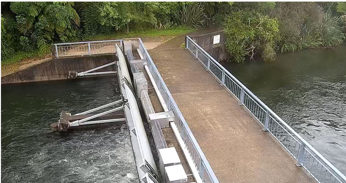
Figure 17 Okere Gates structure fully open to relieve lake levels above consented maximum February 2023
