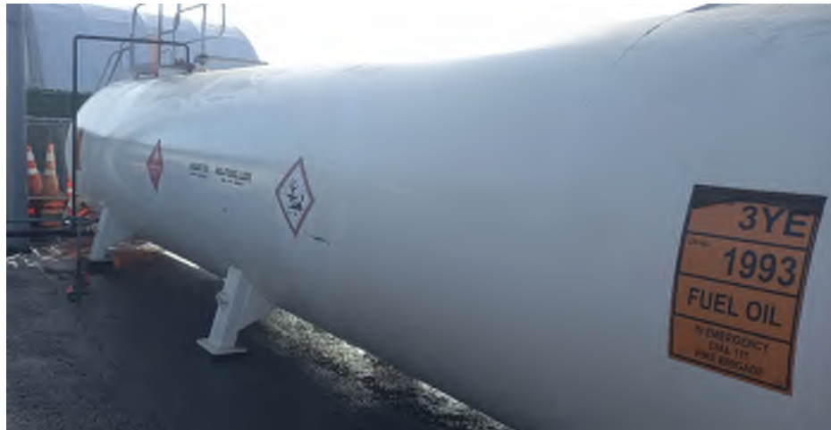
Photo 21: White 50,000 Litre tank containing refined (waste) oil. Located directly outside the site boundary to the east in close proximity to the asphalt plant.
