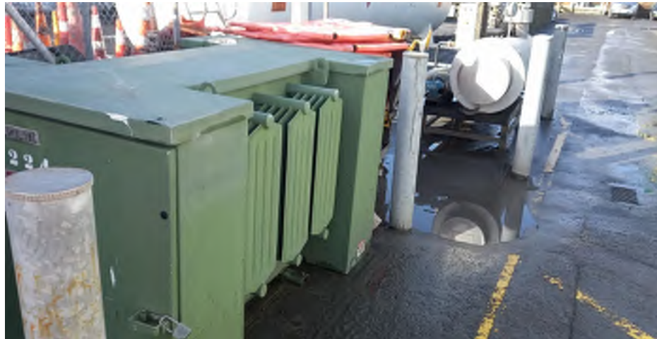
Photo 19: Electrical transformer located on the eastern boundary of the site beside the asphalt plant.
