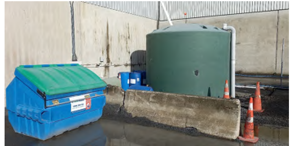
Photo 12: Rainwater tank and skip bin used for site waste such as plastic bags. Storage of 400 L bitumen release behind the water tank.
