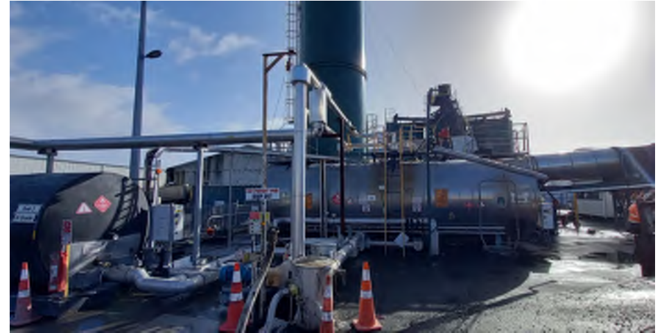
Photo 2: The current asphalt plant located towards the north-eastern corner of the site includes two bitumen storage tanks which are located to the west of the Lime silo.
