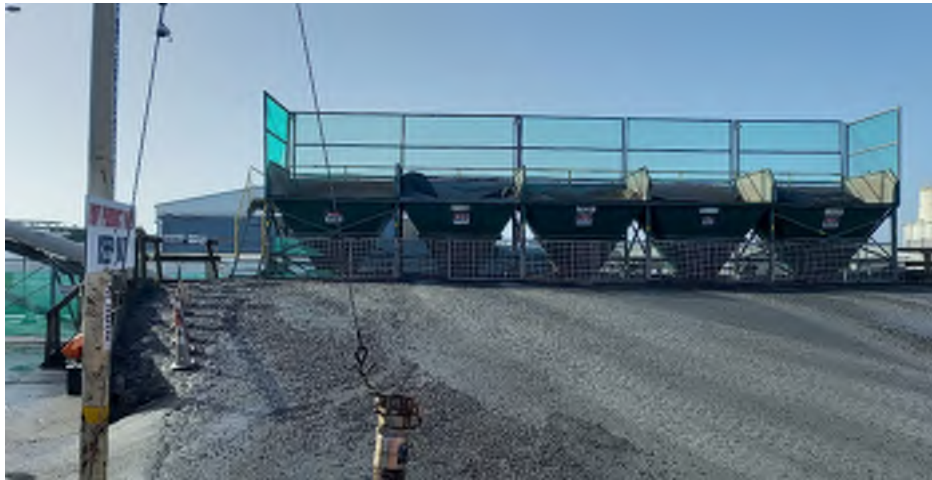
Photo 3: Portable hot storage hoppers and ramp located mid-way along the site's eastern boundary.
