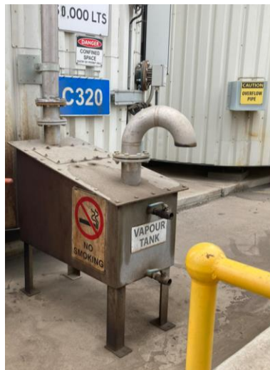
Figure 2.2: Bitumen tank venting waterbath system in place at the Laverton, Australia site Source: Fulton Hogan
