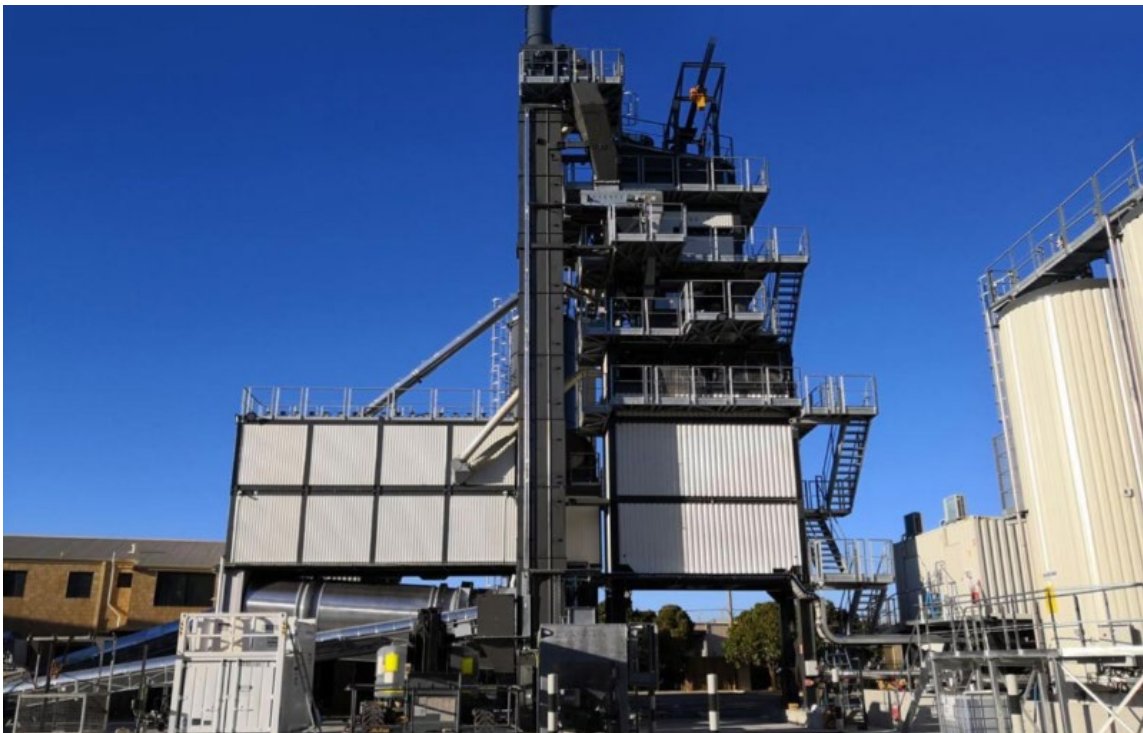
Figure 11: Specimen Asphalt Plant Image
