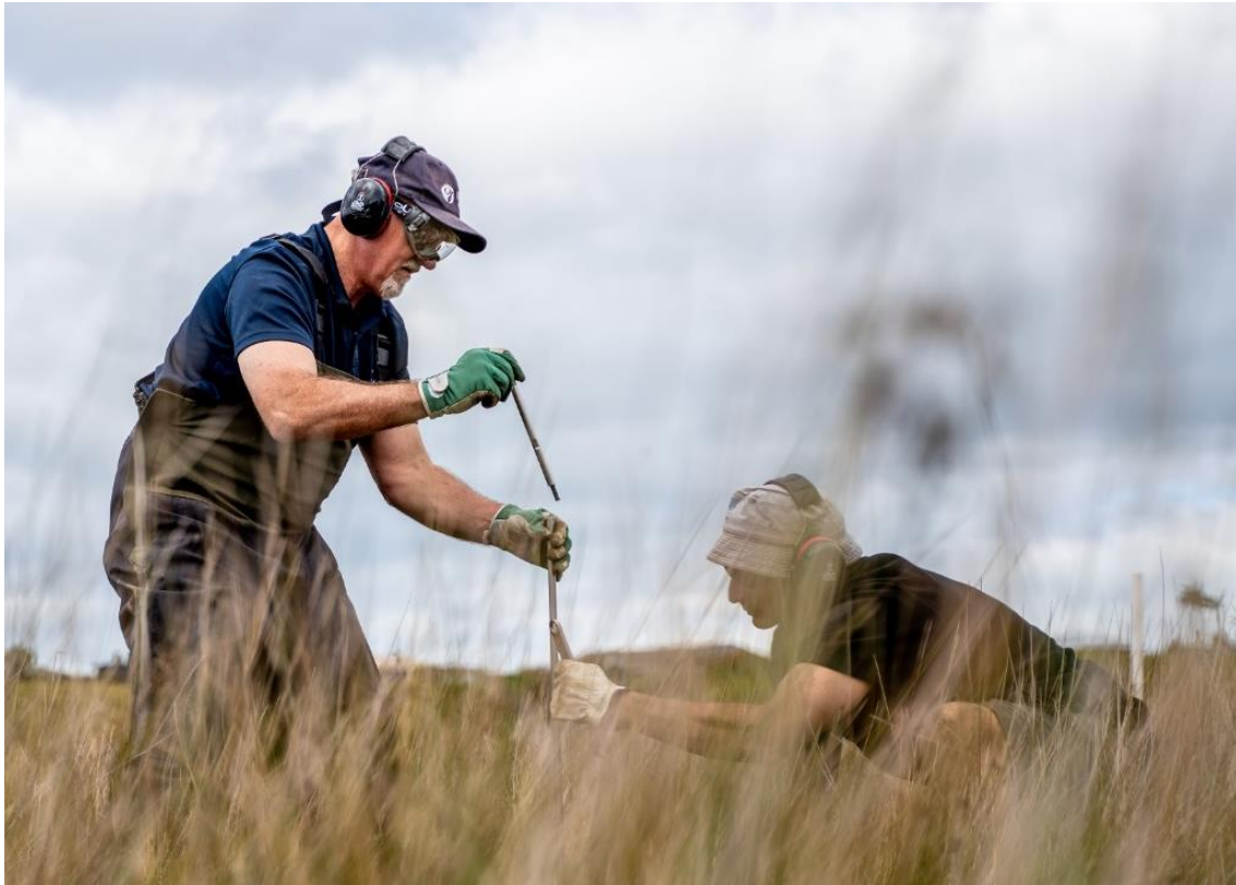
Figure 2-12: RSET Driving head installed to the top of the SS rod before hammering.
