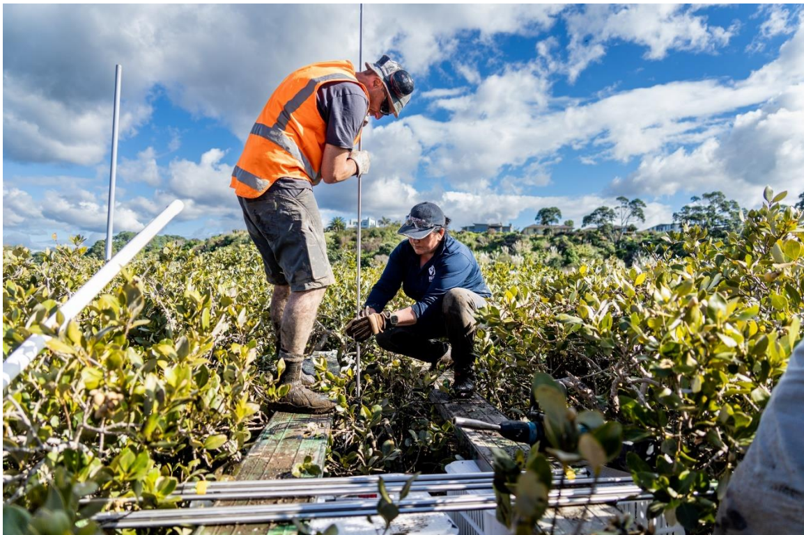
Figure 2-7: Photo of aluminium plank placed either side of the RSET benchmark point during installation. The aluminium planks are 3.0 m in length and supported by plastic baskets or step stools on each side of the no-walk area.
