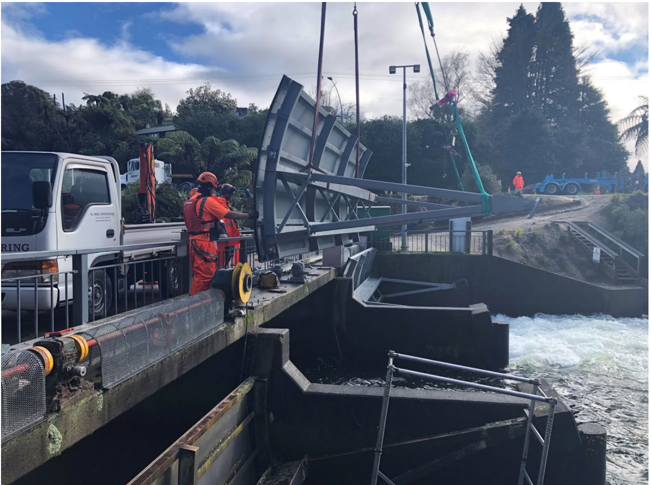
Figure 1 Okere Gates – BOPRC Rivers and Drainage staff and contractors reinstating Gate #2 following scheduled maintenance – May 2020.
