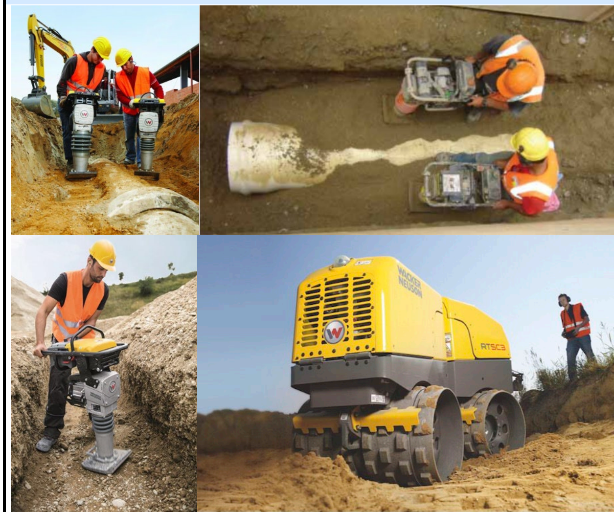
Figure 27 Example of pipe installation with mechanical soil compaction of bedding and surround materials in layers (Photos: Wacker Neuson/Humes)
