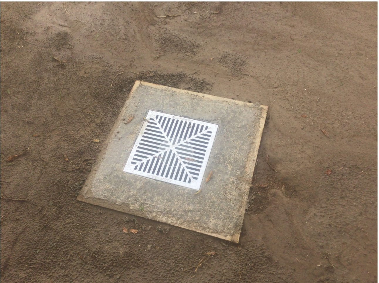
Seepage pressure relief well – allows seepage pressure to be released safely to ground surface (above)
