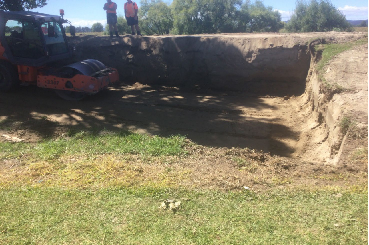
Tree roots excavated and vibrating roller compacting backfill to reinstate stopbank (above)
