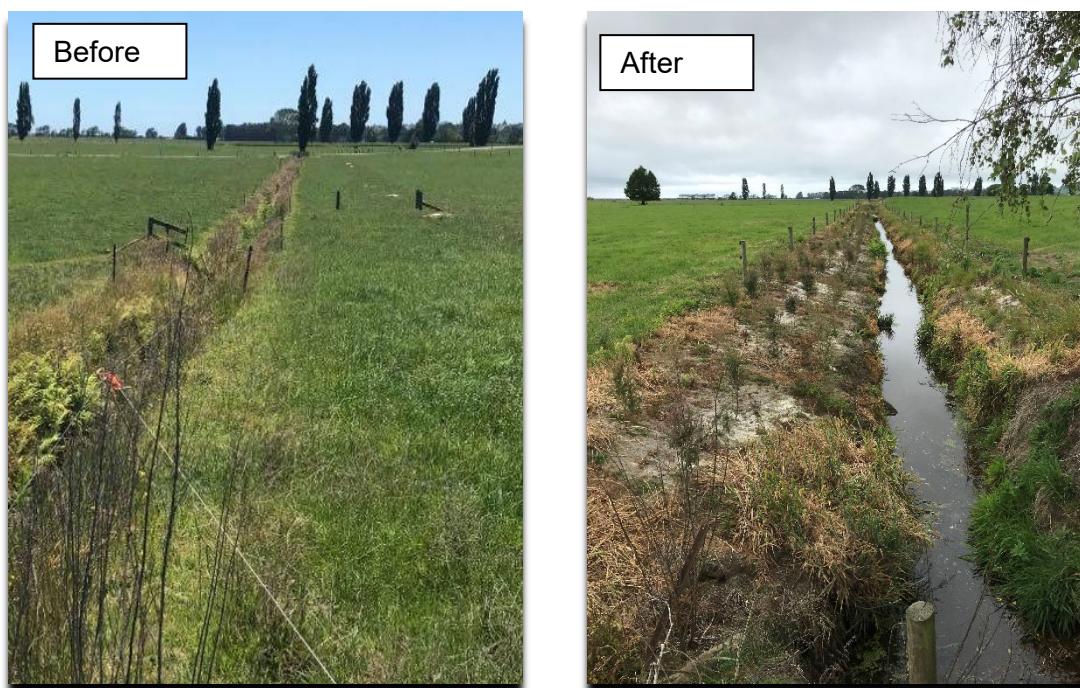
Figure 4: Example of a recently upgraded private farm drain in the Kaituna (Ford Road Focus Catchment).
