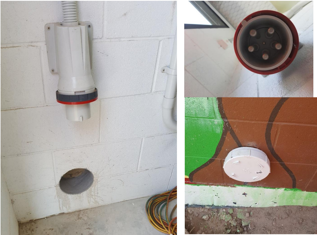
Figure 1 Portable Diesel Generator socket.
