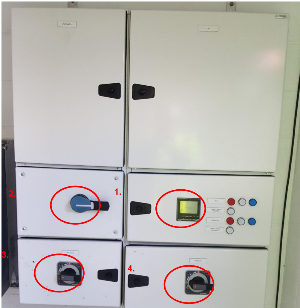
Figure 4 Electrical isolation points – Distribution board
