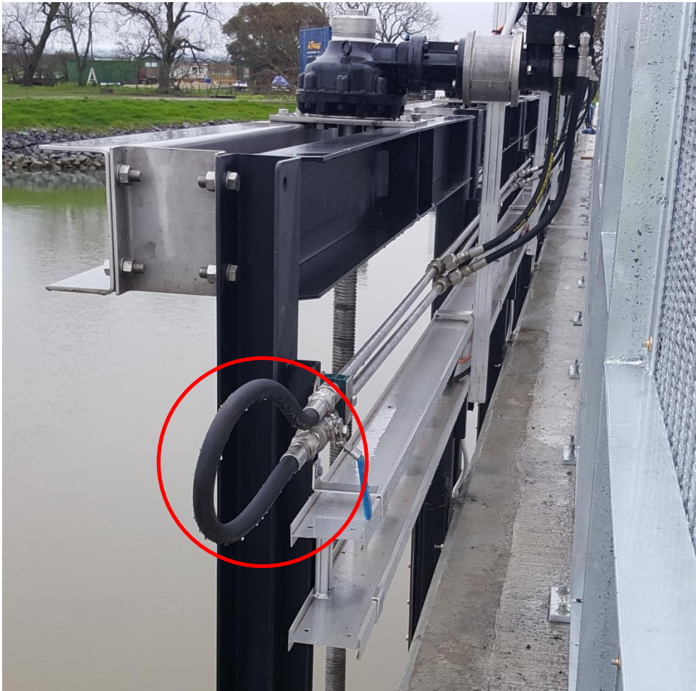
Figure 6 Hydraulic system pressure balancing valve – gate 12
