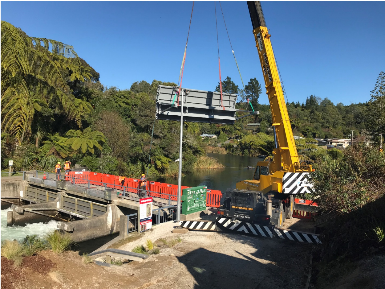
Figure 1 Okere Gates – BOPRC Rivers and Drainage staff and contractors reinstating Gate #1 following scheduled maintenance – May 2020.
