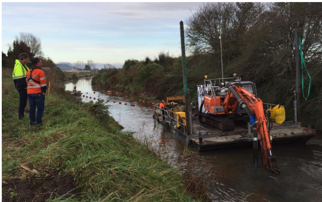
Figure 2. Dredging in section 4 between Paroa Rd and SH30, being observed by independent reviewer and Contractor.
