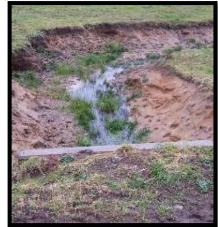
Figure 14 Stormwater Drain Discharging into Waipu Estuary 2013
