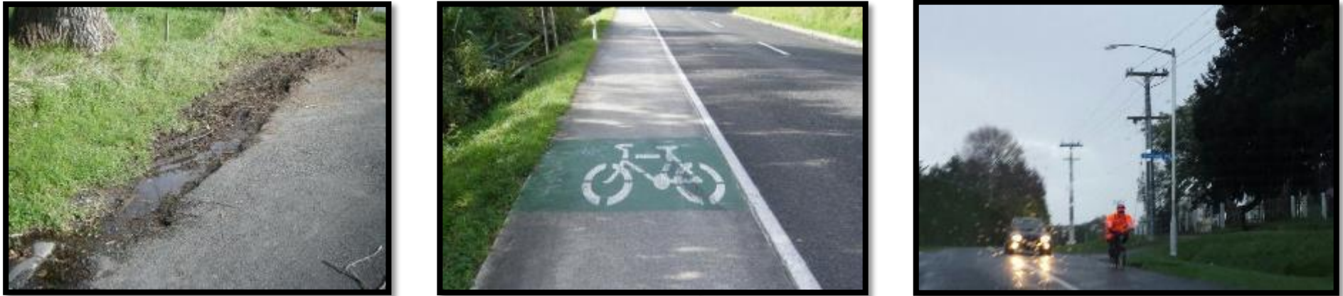
Figure 9 Roadside Impacts Lacking Kerb and Channelling and Cyclist Issue
