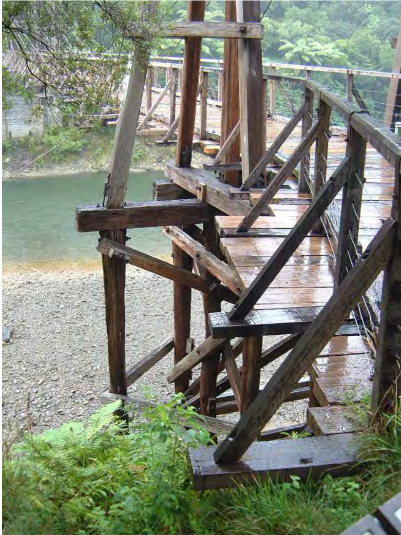
Figure 24 Tauranga Bridge in the Waioeka Gorge is a variation on conventional suspension bridges, which originated in early 19th century England. The 'harp' bridge is rare in New Zealand.
