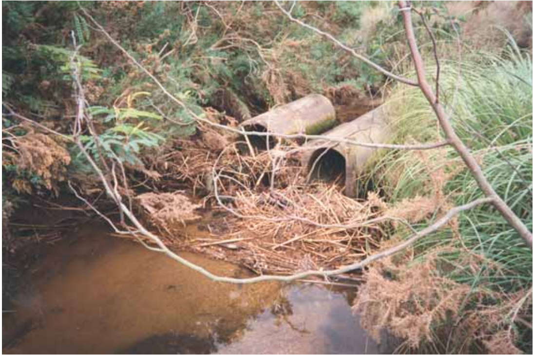
Figure 13.9 Culverts collect debris, and partially block the flow.
