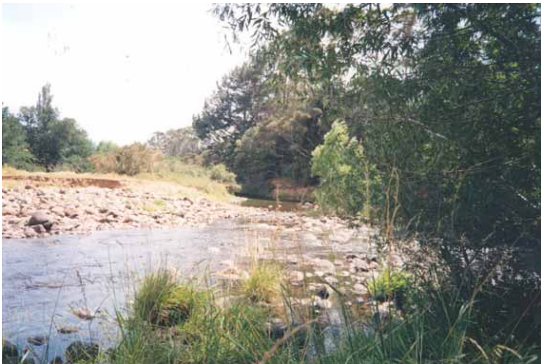
Figure 24.8 Minor erosion of the left bank at 2.6km.
