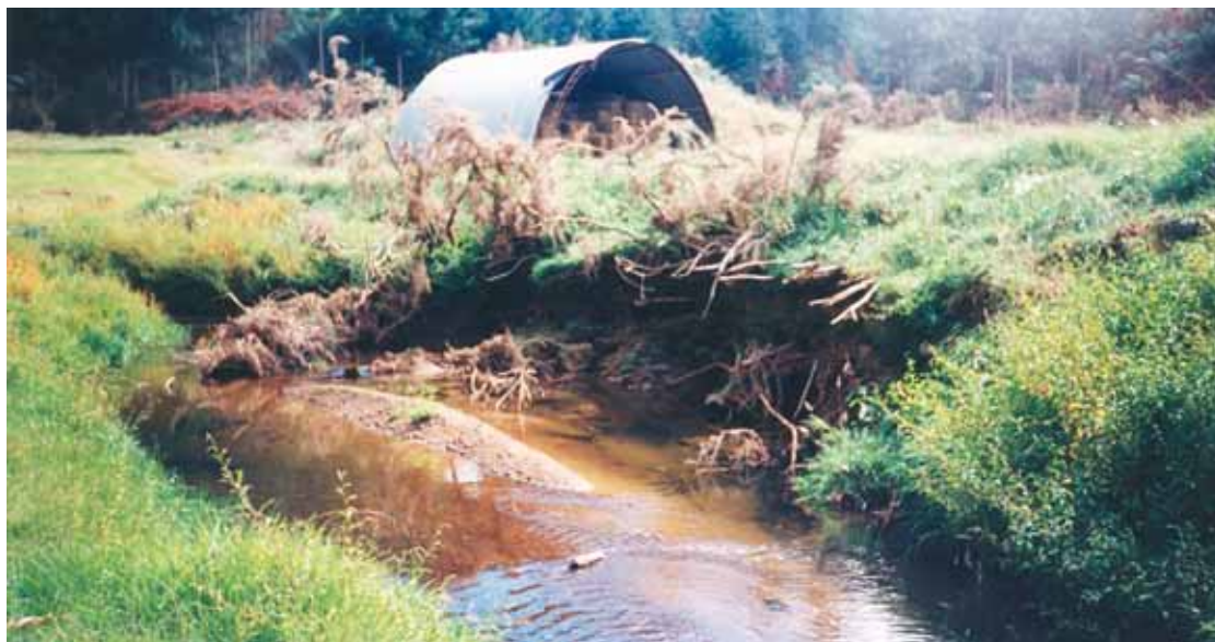
Figure 3.7 An eroding stopbank at 3.45km
