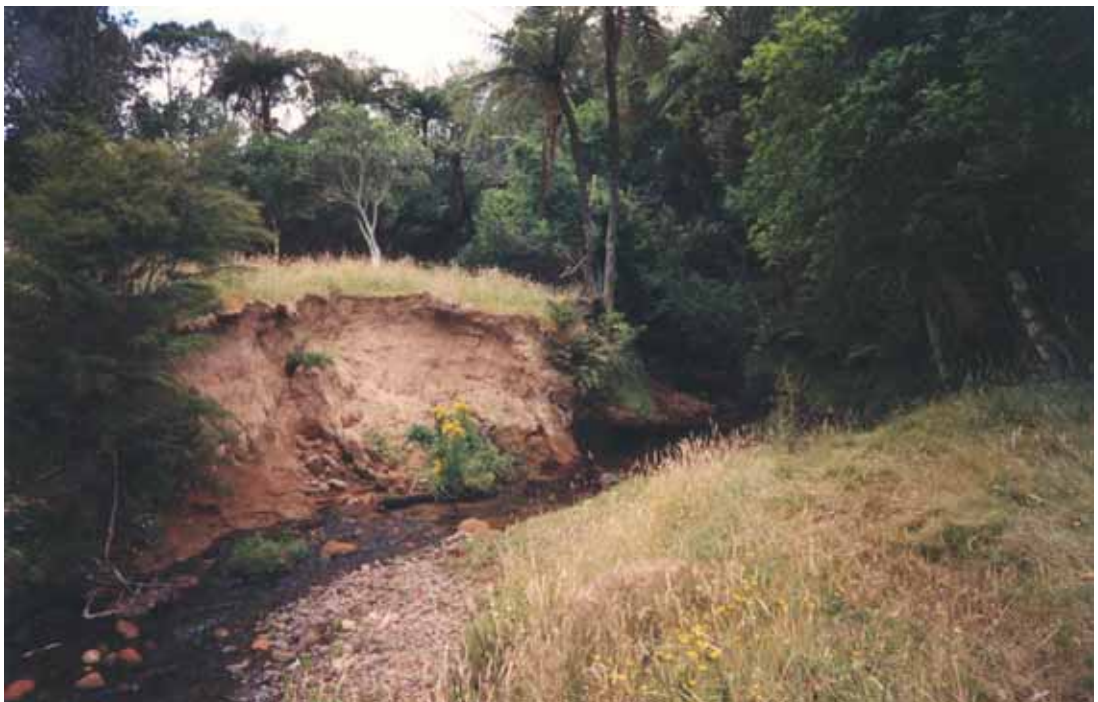
Figure 20.2 Erosion of the left bank at 4km above SH2. Downstream of this banks continue to erode in approximately 5m lengths in the open areas.
