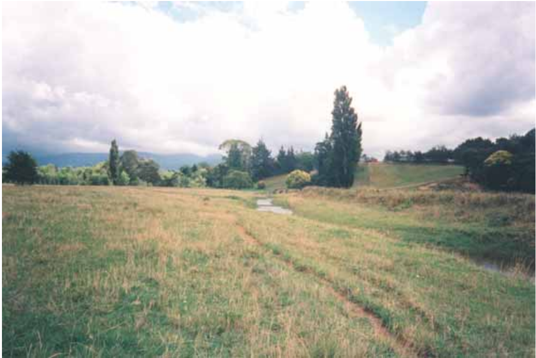
Figure 18.8 Upstream view at 800m of an open floodplain with grasses to the waters edge. The stopbank on the true left is in good condition.
