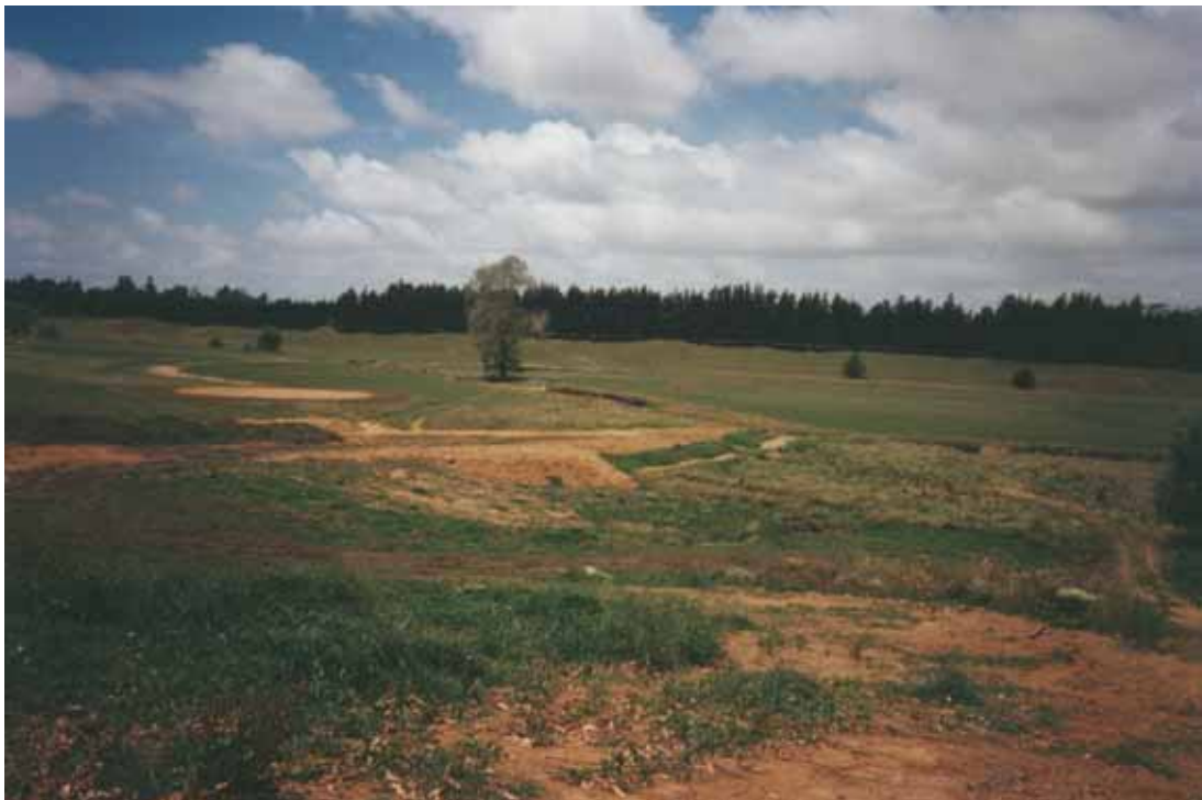
Figure 18.9 Construction work is underway at 1.3km. Heavy vehicle tracks are present down to the streams edge.
