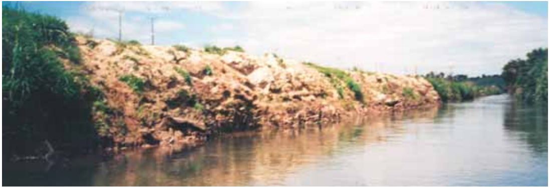
Figure 7.3 Dumped fill adjacent to stream has not yet been tested by flood flows.
