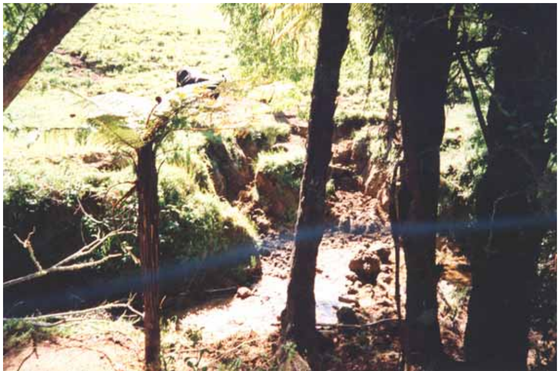
Figure 13.1 Slumping of the right bank at 5.0km.
