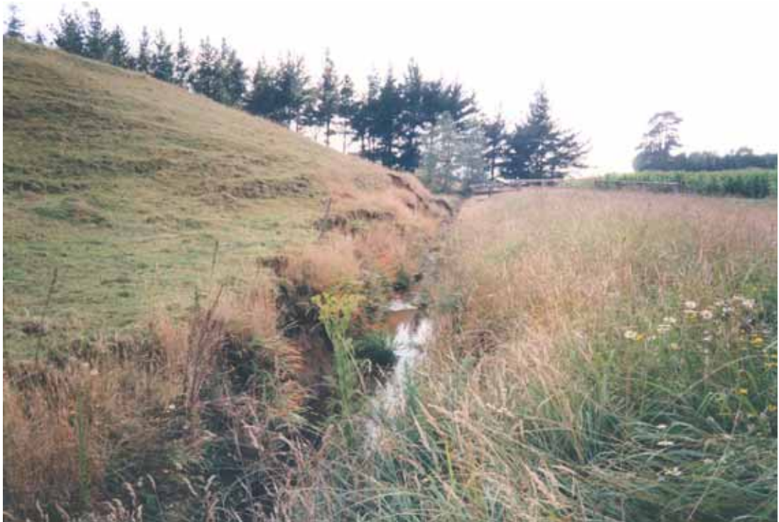
Figure 23.6 Bank erosion at 1.3km.
