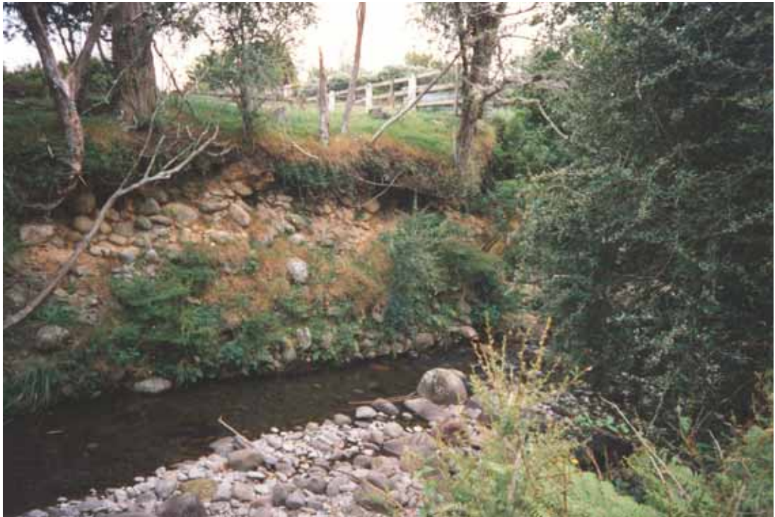
Figure 16.3 Previous undermining of the right bank exposes tree roots. The lower bank remains well vegetated.
