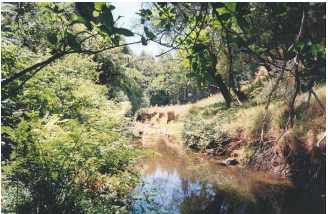
Figure 22.8 Erosion of the right bank where thick bank vegetation is absent.
