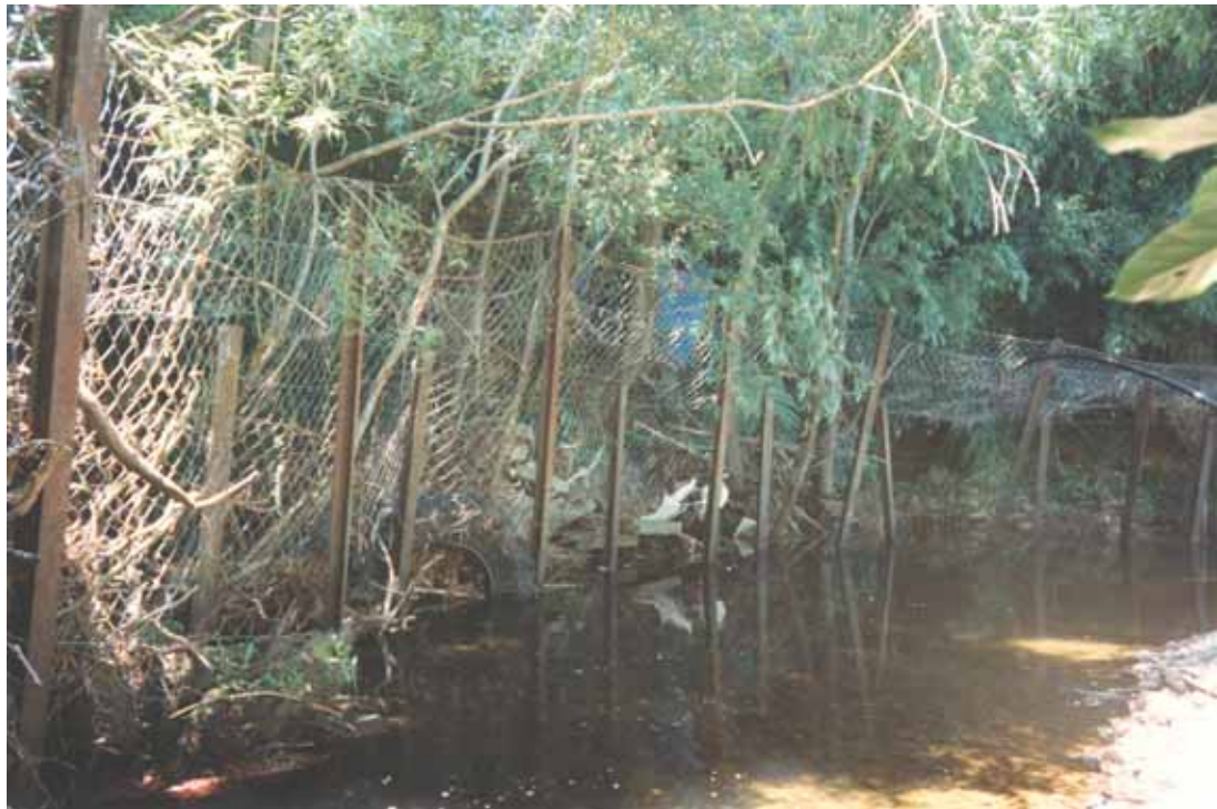
Figure 18.5 Fencing along the left bank holds back trees, rubbish and other debris.
