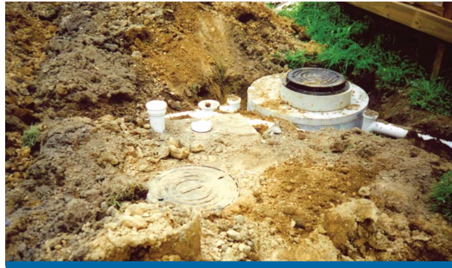
A septic tank system.
