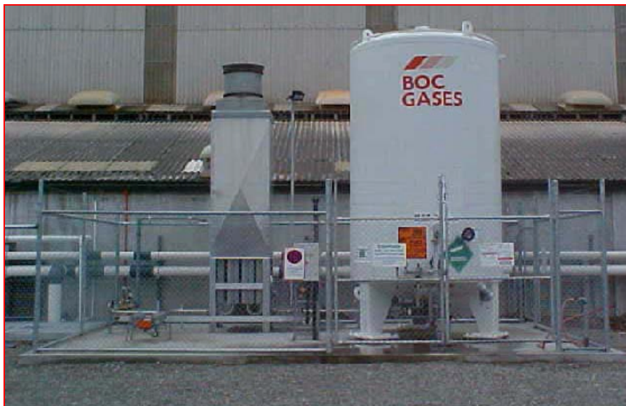
Figure 4: A typical BOC onshore oxygen installation
