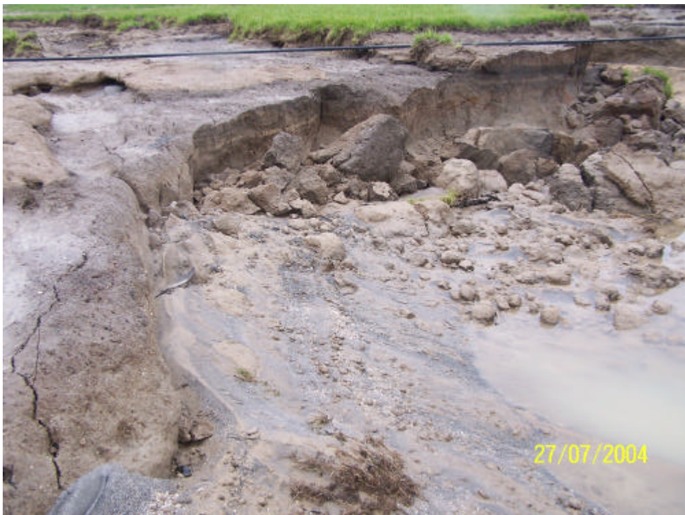
Photograph 7: Cracking and collapse of slightly cohesive upper soil layers at the far end of the scour hole
