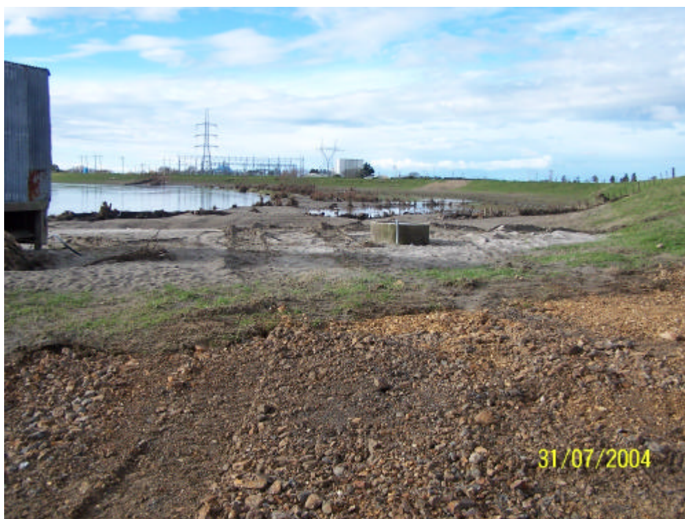
Photograph 8: Pump shed and river berm
