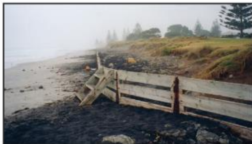
December 1998 The dilapidated and non-functional seawall. Note erosion on the landward 'protected' side.
