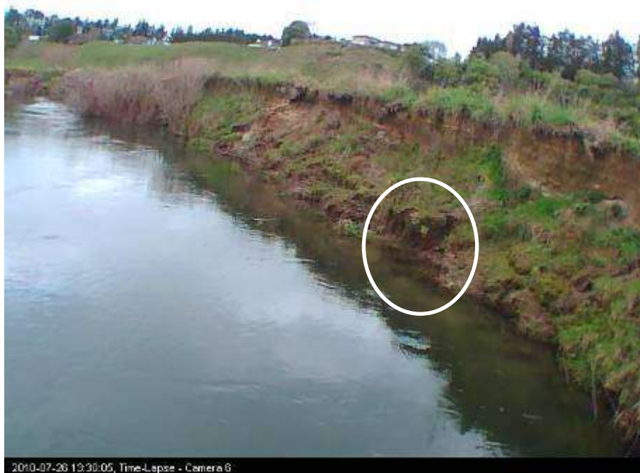
Figure 3-69: Final photograph at Site 6 taken on 26/7/10. The area circled highlights an area of bank erosion since the start of surveillance.
