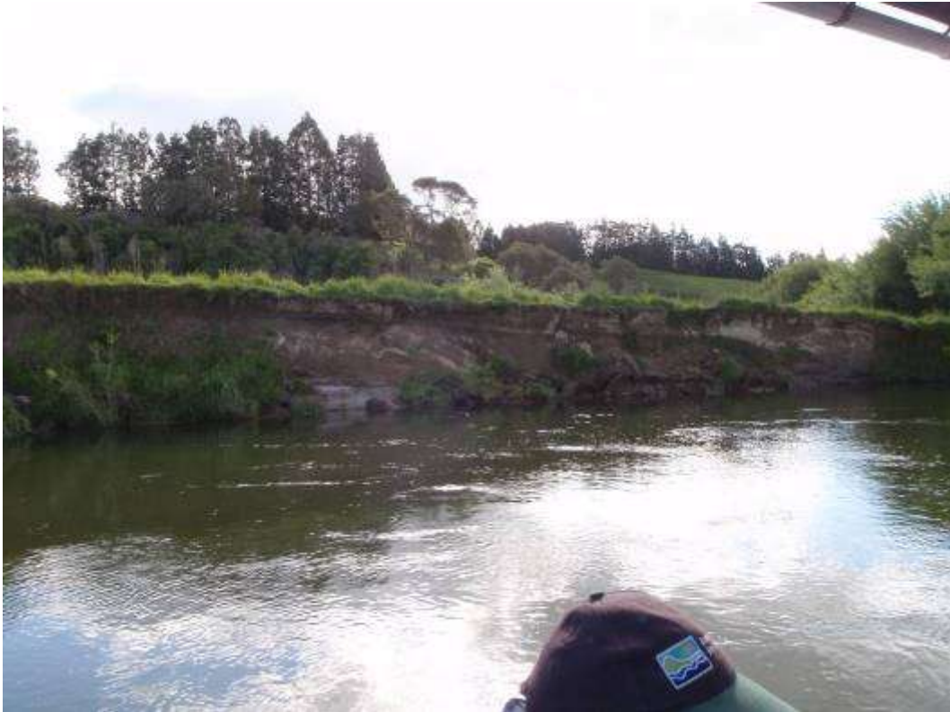
Figure 2-6: Bank erosion Site 6. Located at E2808166 N63670551 on the left bank of the control reach.
