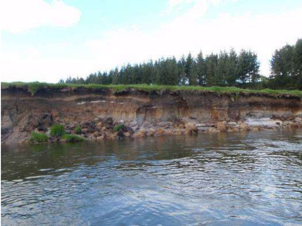
Figure 2-7: Bank erosion Site 7. Located at E2807956 N6370912 on the right bank of the control reach.
