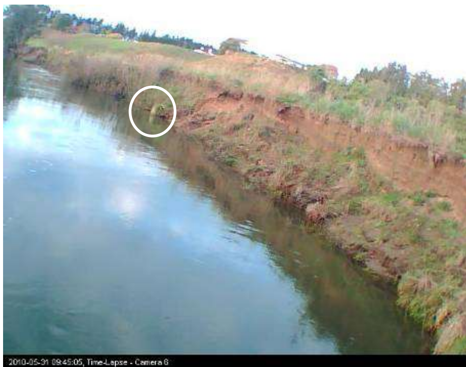
Figure 3-67:Site 6 after floodwaters had receded on 31/5/10. Circled feature to be compared with photo prior to flood.
