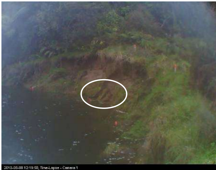
Figure 3-26: Active erosion at waters edge at Site 1 on 8/8/10 at 12:20. See the following figure for the same site 5 mins later.
