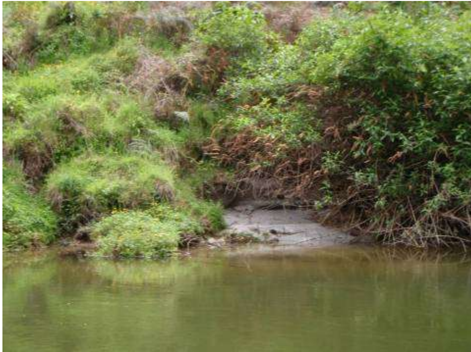
Figure 1-3: Typical 'slump' type of erosion. The same type of erosion was recorded at this site in 2004. This slump extends at least 15 m up the bank.
