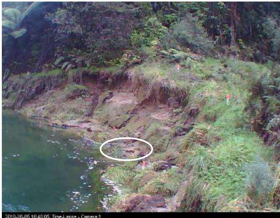
Figure 3-18: Active erosion at waters edge at Site 1 on 5/6/10. See following figure for site 10 mins later.
