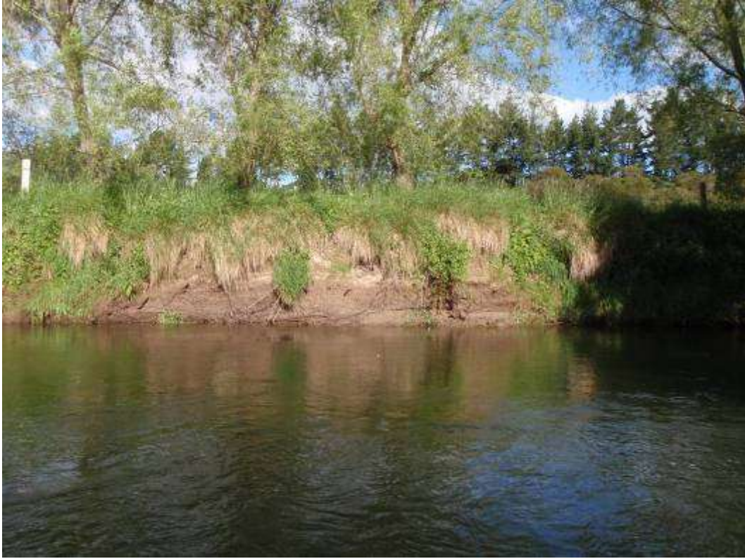
Figure 2-5: Bank erosion Site 5. Located at E2808574 N6370097 on the right bank of the control reach.
