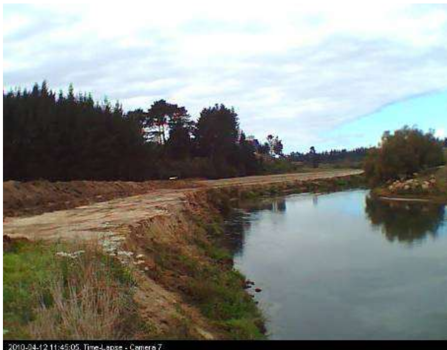
Figure 3-72:Site 7 part way through battering of the bank on 12/4/10. Note cows on opposite bank.
