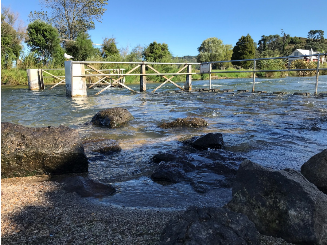
Figure 9 Ohau Weir fish pass during low lake levels in Lake Rotorua
