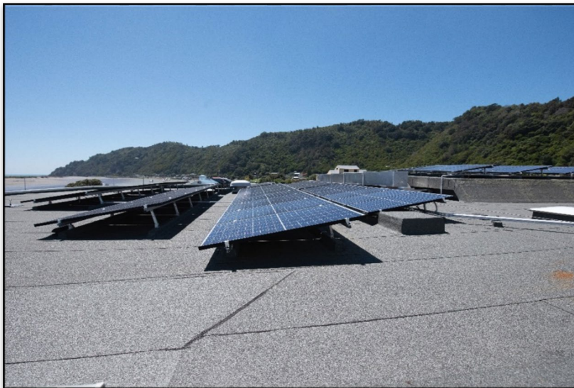
Image 3 Photovoltaic tiles at Offices – 5-11 Quay Street, Whakatāne.
