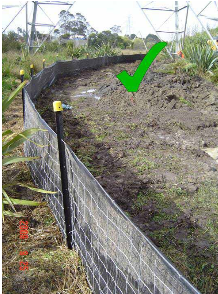
Figure 77 Super silt fence example showing well constructed fence - photo courtesy of Ridley Dunphy Environmental Limited.
