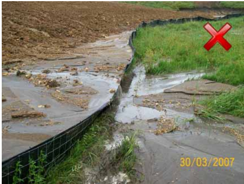
Figure 78 Super silt fence no upslope water control (maintenance required) - photo courtesy of Environment Bay of Plenty.
