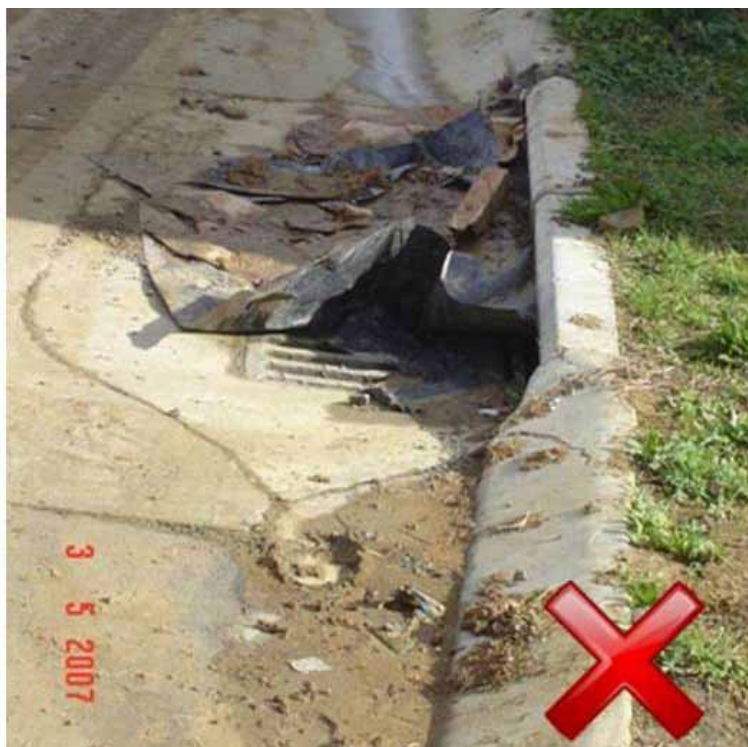
Figure 90 Storm water inlet fully blocked leading to downstream flooding - Photo courtesy of Ridley Dunphy Environmental Limited.
