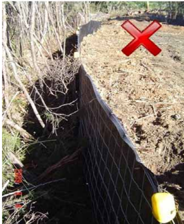
Figure 74 Super silt fence used to retain material - photo courtesy of Ridley Dunphy Environmental Limited.
