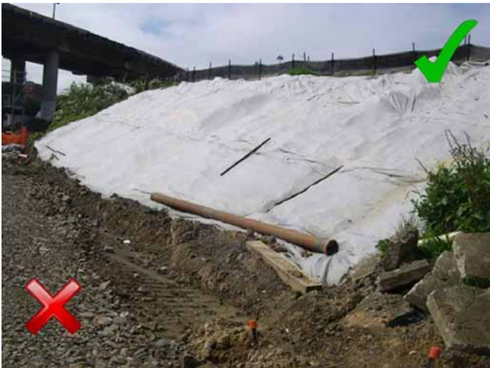
Figure 19 Geotextile showing overlap and top key support. Not appropriately pinned to slope - photo courtesy of Ridley Dunphy Environmental Limited.
