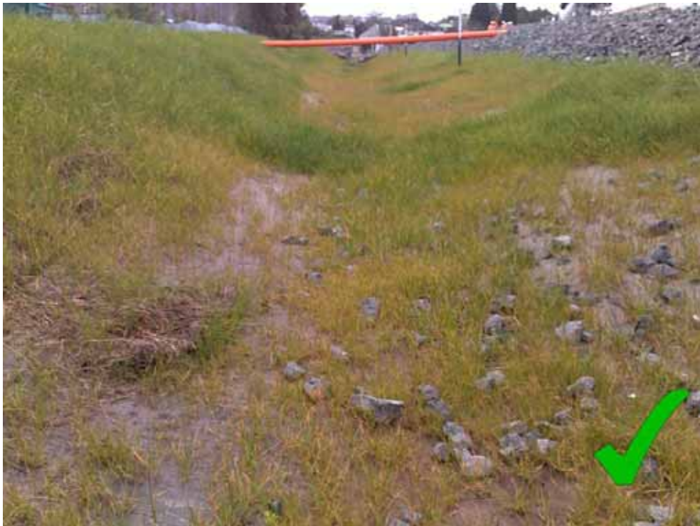
Figure 21 Matting utilised to assist with vegetation establishment in channel – photo courtesy of Ridley Dunphy Environmental Limited.
