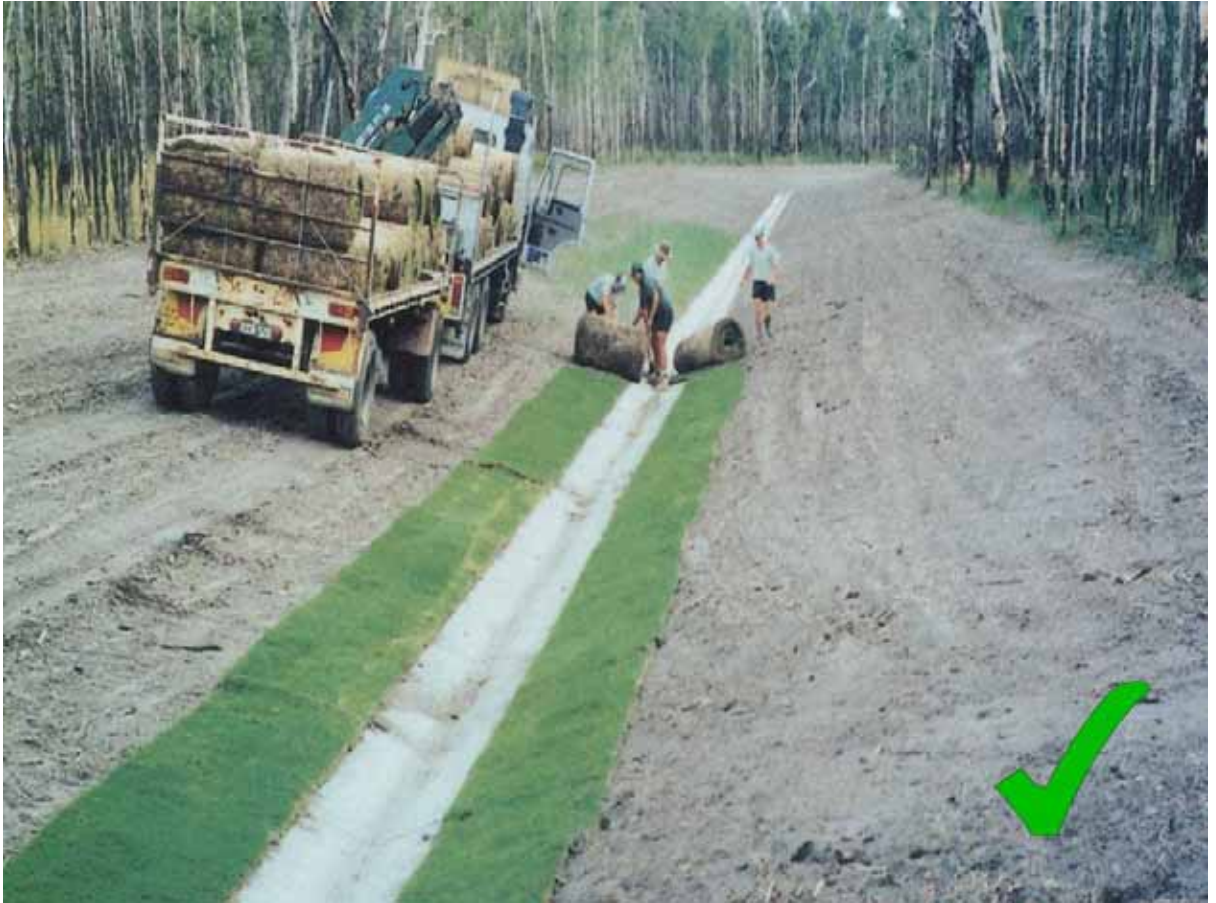
Figure 17 Laying turf next to drainage channel - photo courtesy of Auckland Regional Council.
