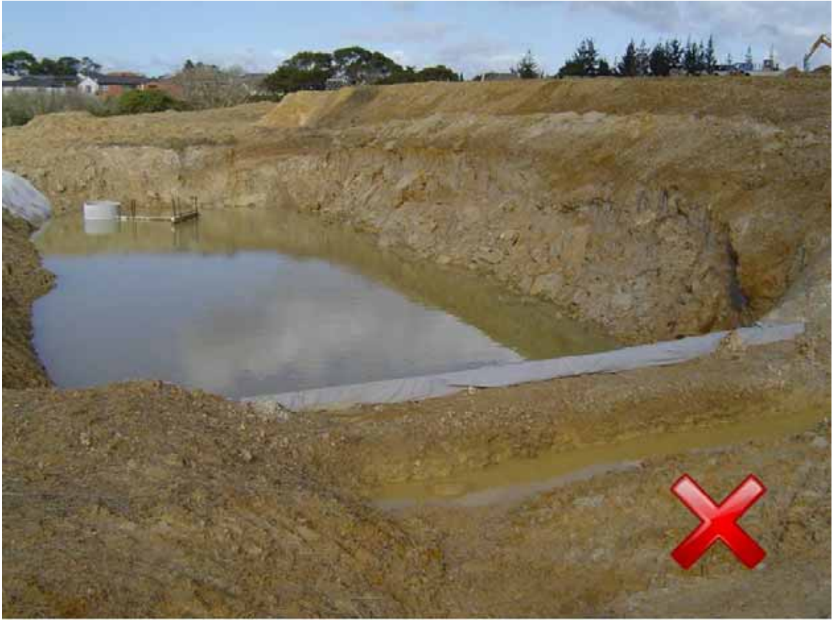
Figure 58 Collapsing sediment retention pond embankment - Courtesy of Ridley Dunphy Environmental Limited.
