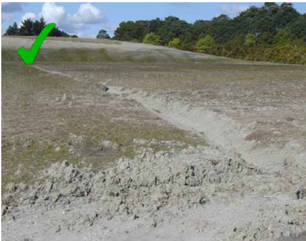
Figure 25 Contour drain - photo courtesy of Ridley Dunphy Environmental Limited (Note that contour drain base could be better shaped to avoid erosion).
