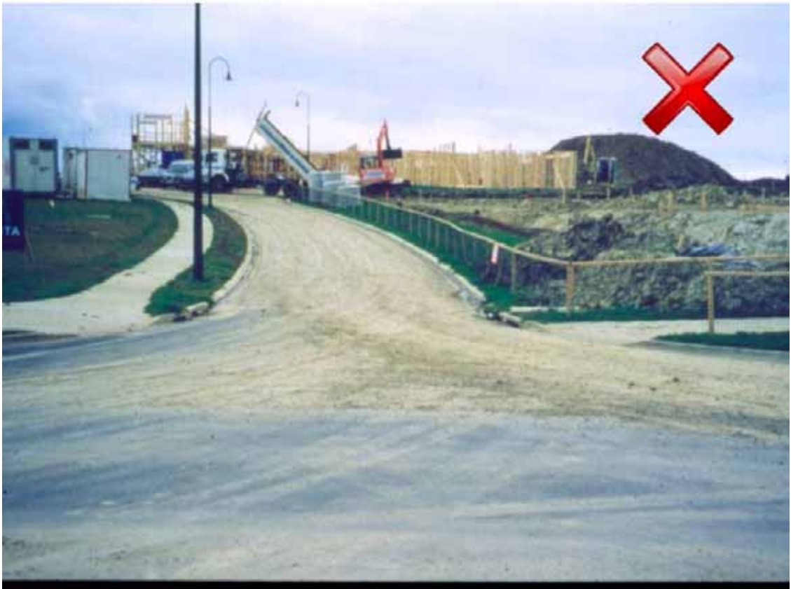
Figure 44 Sediment on road – no stabilised entrance way - photo source unknown.
