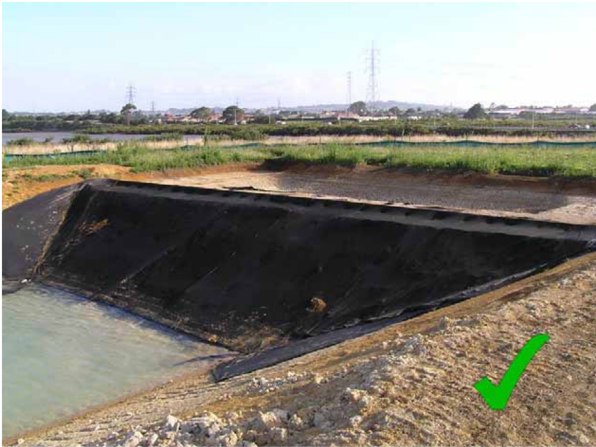
Figure 53 Forebay and level spreader - courtesy of Environment Waikato.
