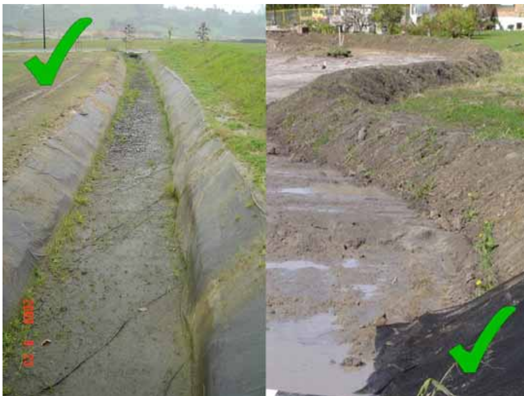
Figure 28 Clean water diversion channel diverting water away from site (on left) and dirty water diversion channel directing sediment flows to retention structure (on right). Photos courtesy of Ridley Dunphy Environmental Limited.
