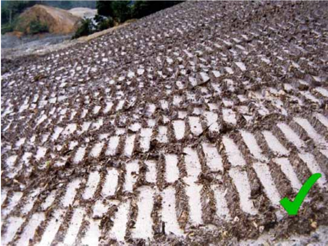
Figure 48 Slope with surface roughening undertaken. Note the fine grained-sediment caught in the hollowed areas behind the mounds caused by the tracks. These have acted as micro sediment traps - photo courtesy of Auckland Regional Council.
