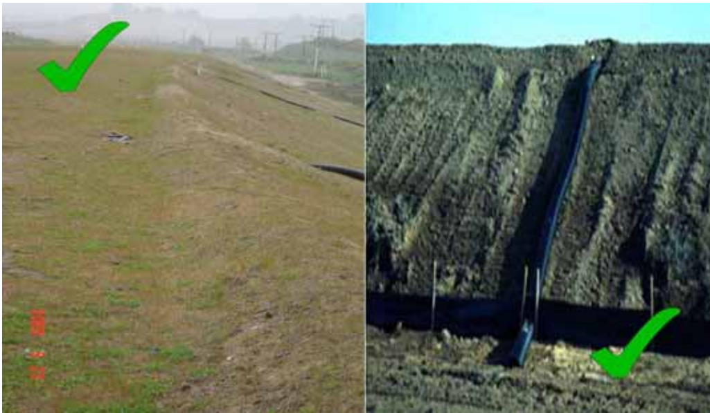
Figure 36 Diversion channel leading to structure and pipe taking flows down slope - photos courtesy of Ridley Dunphy Environmental Limited.
