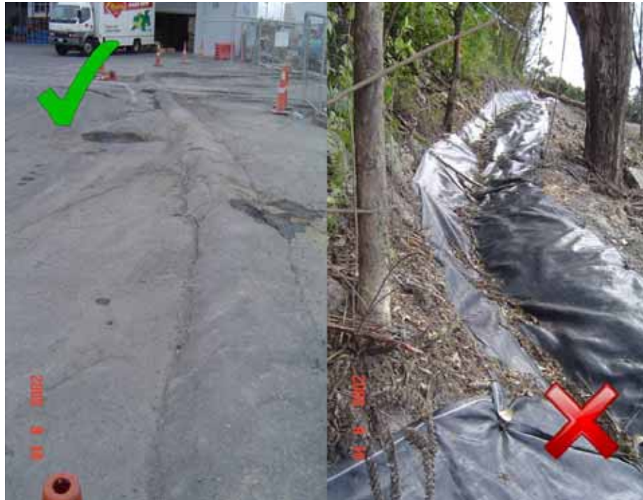
Figure 31 Good asphalt clean water diversion and bad geotextile example - photos courtesy of Ridley Dunphy Environmental Limited.
