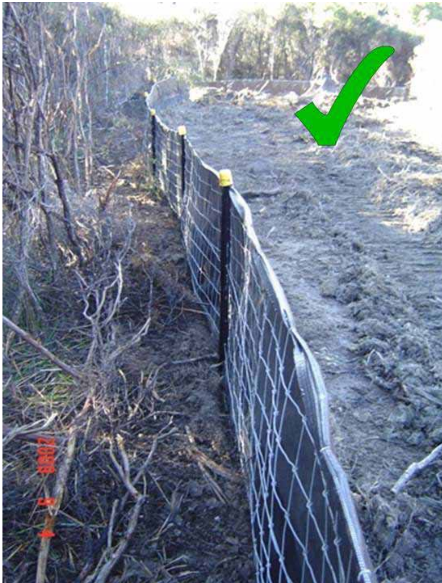
Figure 75 Super silt fence clearly delineating disturbed area and protected vegetation - photo courtesy of Ridley Dunphy Environmental Limited.
