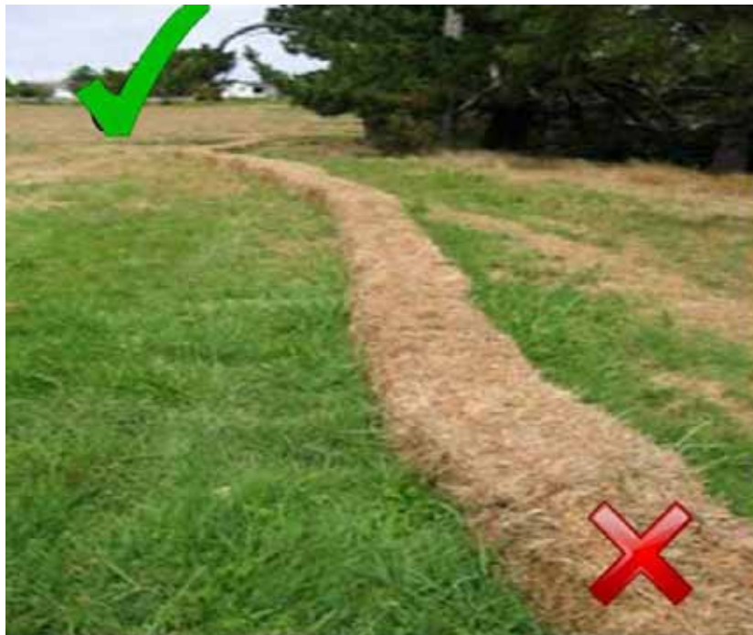
Figure 86 Hay bale barrier – on contour however placed wrong way with no stakes - photos courtesy of Environment Canterbury.
