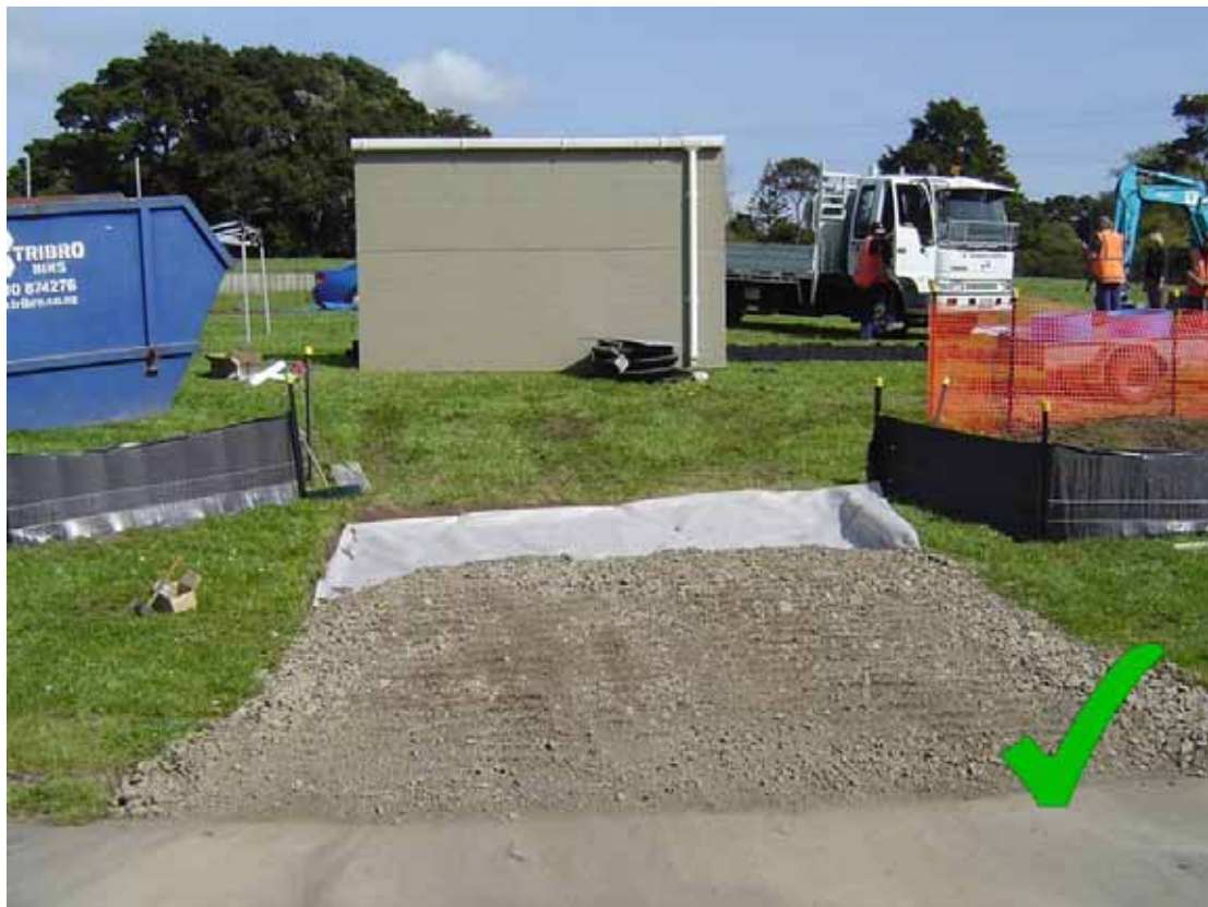
Figure 45 Stabilised entrance way as part of a small site development – photo courtesy of Auckland Regional Council.
