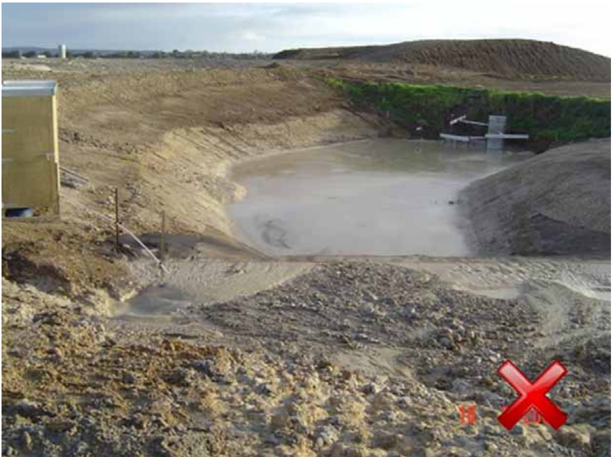
Figure 60 Sediment retention pond forebay requiring maintenance - courtesy of Ridley Dunphy Environmental Limited.
