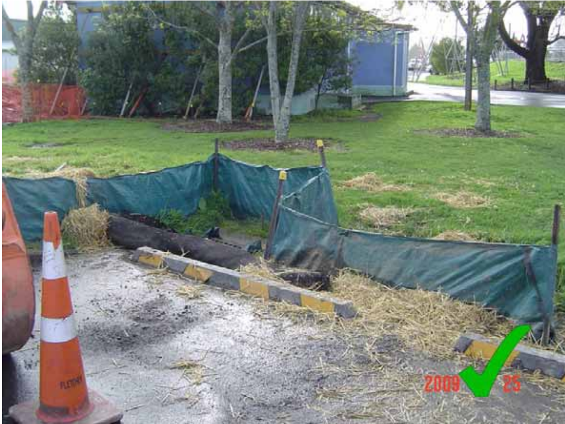
Figure 89 Storm water inlet protection (filter media with silt fence protection from grass/disturbed surface) - photo courtesy of Ridley Dunphy Environmental Limited.
