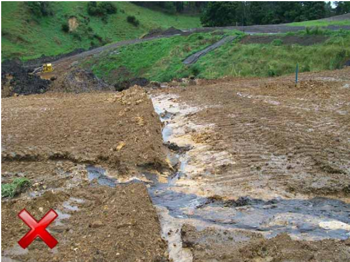
Figure 26 Contour drain – overtopping and short-circuiting of contour drain has reduced its water control ability - photo courtesy of Environment Bay of Plenty
