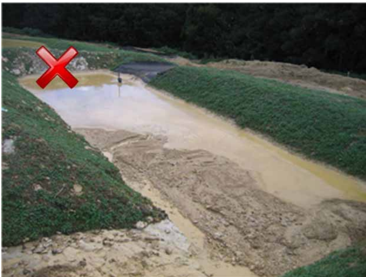
Figure 70 Decanting earth bund which needs maintenance (removal of accumulated sediment) otherwise good length:width ratio and appropriate decant. Photo courtesy of Auckland Regional Council.
