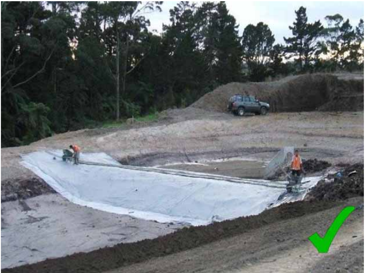
Figure 56 Installation of level spreader and concrete haunching - Courtesy of HEB Construction Limited.
