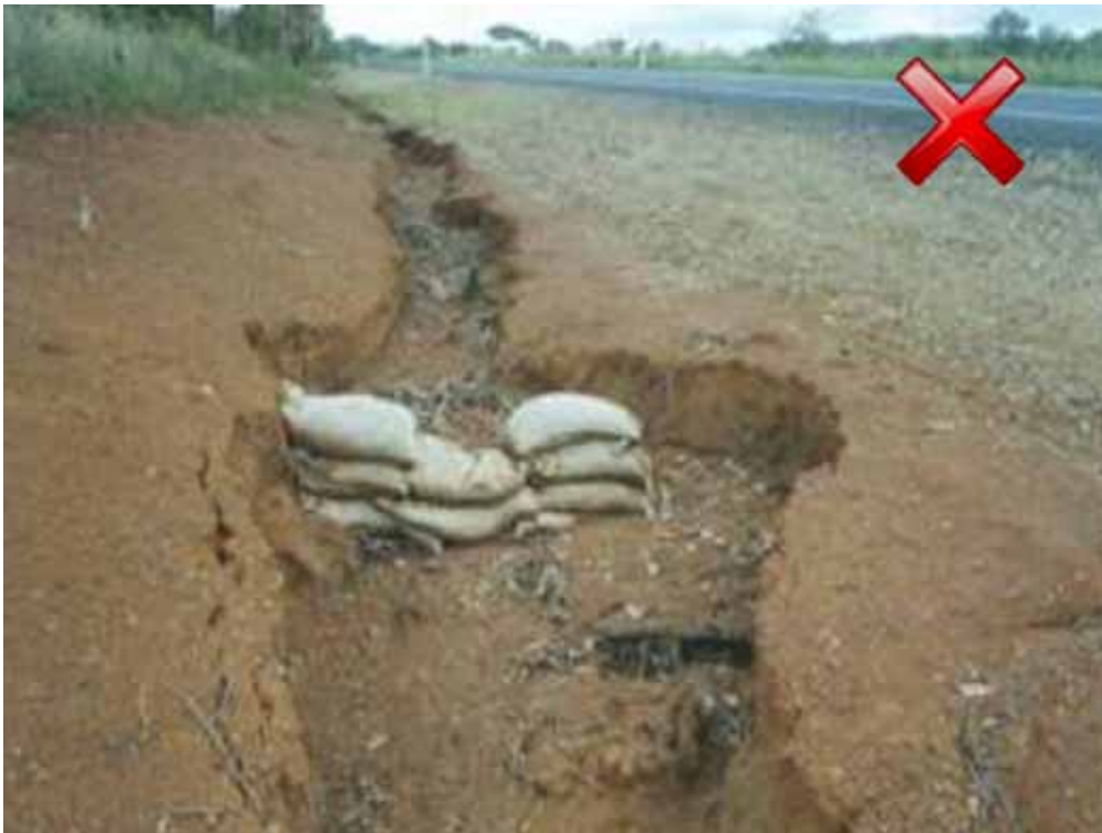
Figure 41 Check dam in highly erodible soils. Problems with excessive spacing, unsuitable location and insufficient up turn resulting in water outflanking the structure - photo courtesy of Environment Canterbury.
