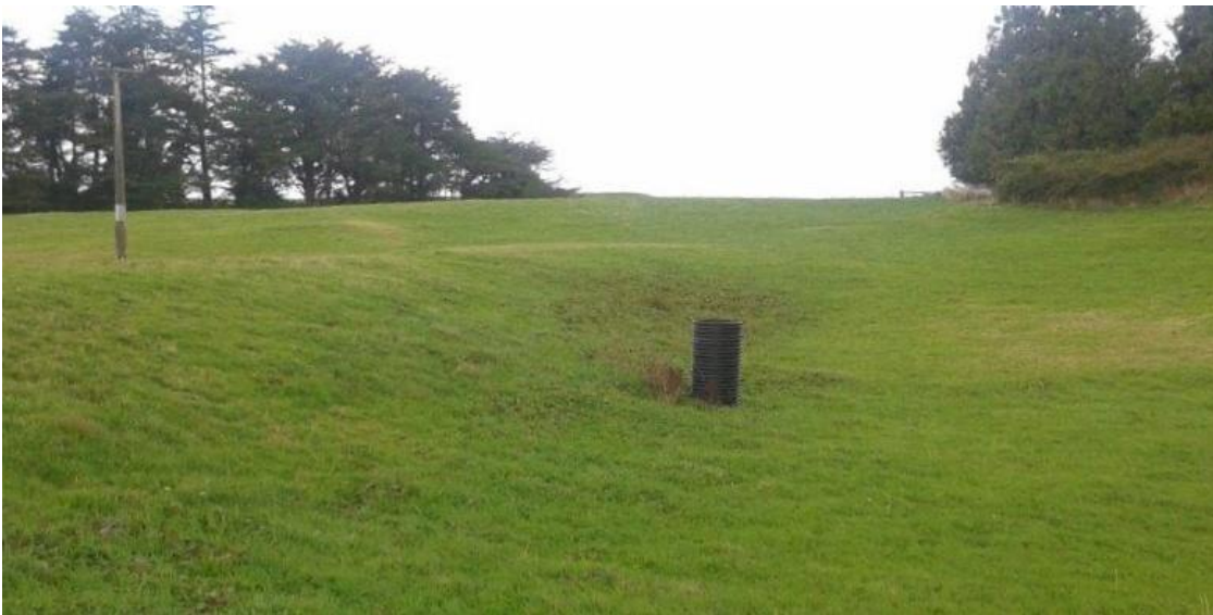
Figure 2.2: Photo of an upstand riser installed in the ponding area of a detention bund. The riser is connected to an outlet pipe that passes through the bund, which discharges ponded runoff on the downstream side.
