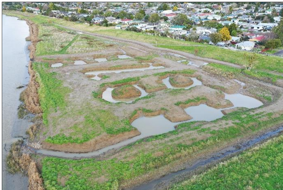
Photo 1: Inanga pond creation on the true right hand side of the Whakatāne River; July 2020
