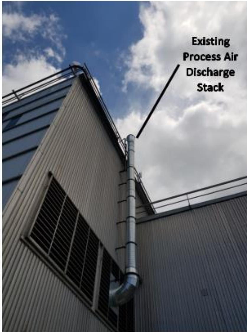
Figure 4 Process Air Discharge Stack
