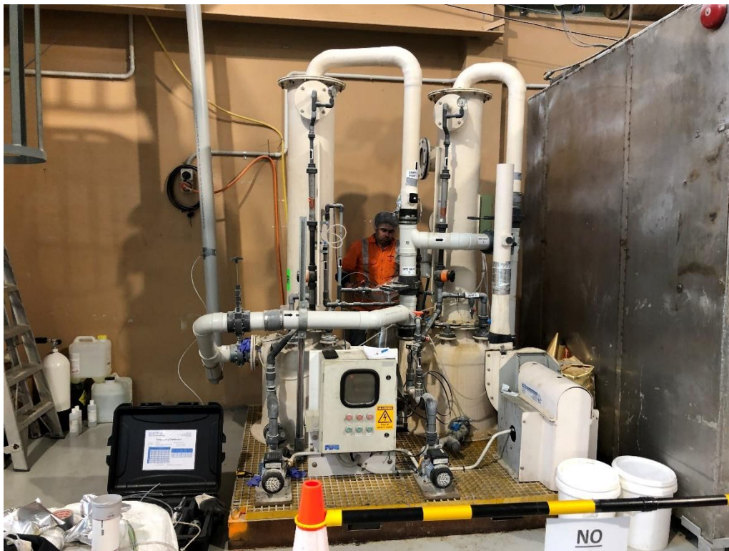
Figure 12 Pilot Plant Scrubber
