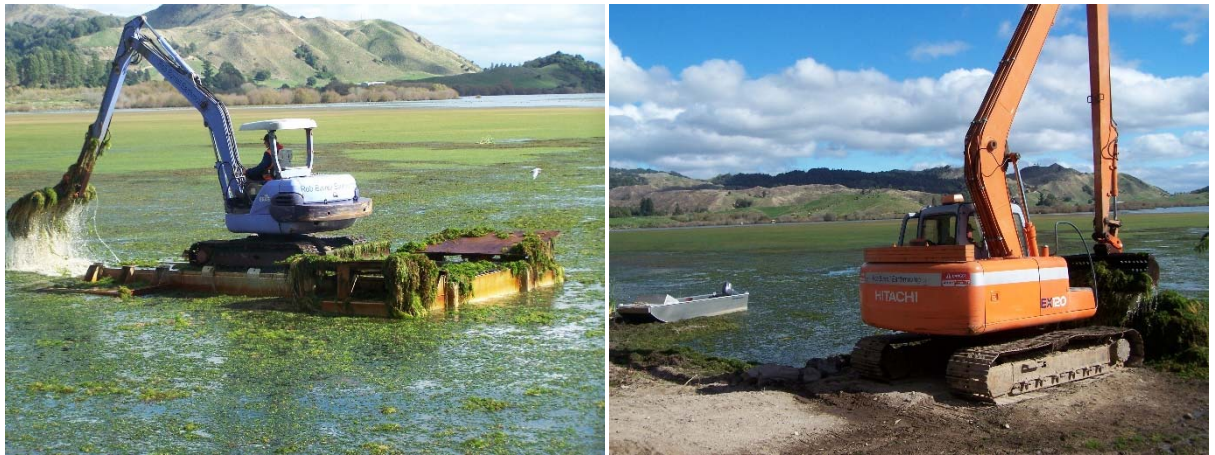
Figure 6 Weed harvesting on Lake Rotoehu in 2013 carried out by Rob Burrell Earthmoving Limited. Two excavators were used (shown in pictures), one a barge on the lake (left) and a long reach machine operated on the shoreline transferring the weed to a truck for removal.
