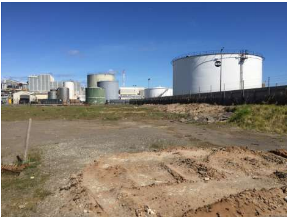
Photo 19 Thin polymer applied to unsealed areas [CMA site, Totara Street, 10:42 AM 18 Oct 2016]
