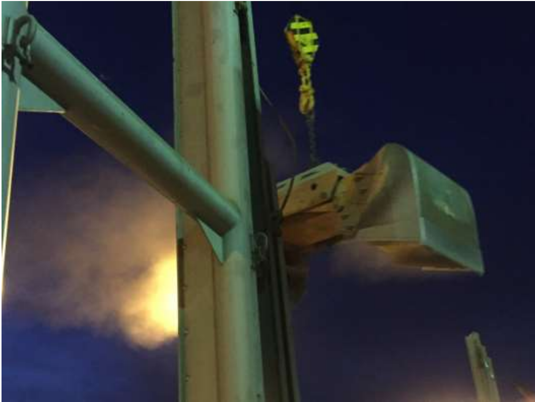
Photo 6 Dust trailing behind grab during clinker unloading [Mount Maunganui Wharves 5:42 AM 21 Oct 2016]
