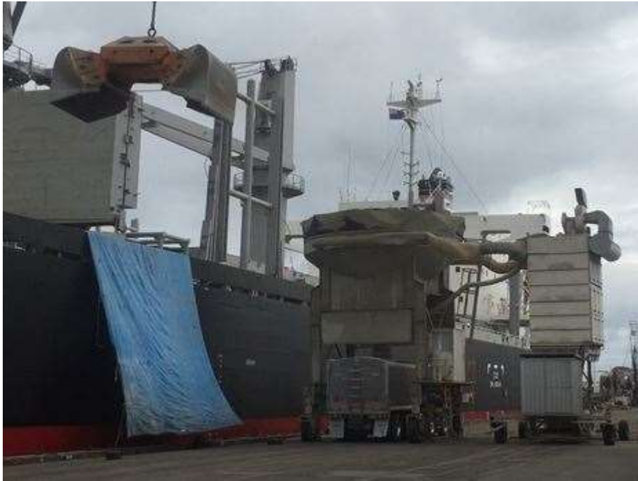
Photo 22 Tarpaulin under path of crane grab during unloading of clinker. [Mt Maunganui Wharves, 11:46 AM 20 Oct 2016]
