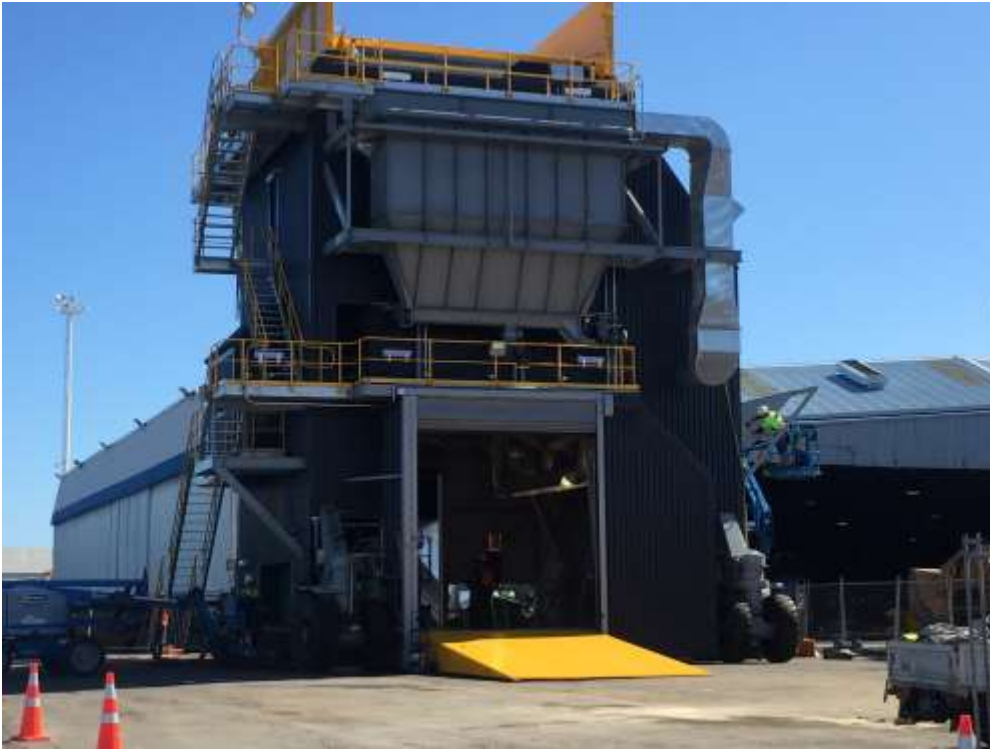
Photo 23 Dedicated hopper with inbuilt extraction and bag filter under construction at Mt Maunganui wharves [Mount Maunganui wharves 10:01 AM 18 Oct 2016]
