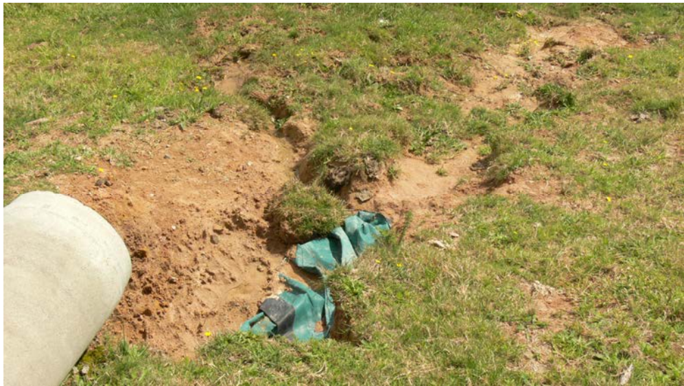
Figure 8: Eroding scarp and drains on road margin in lower Waipapa catchment.
