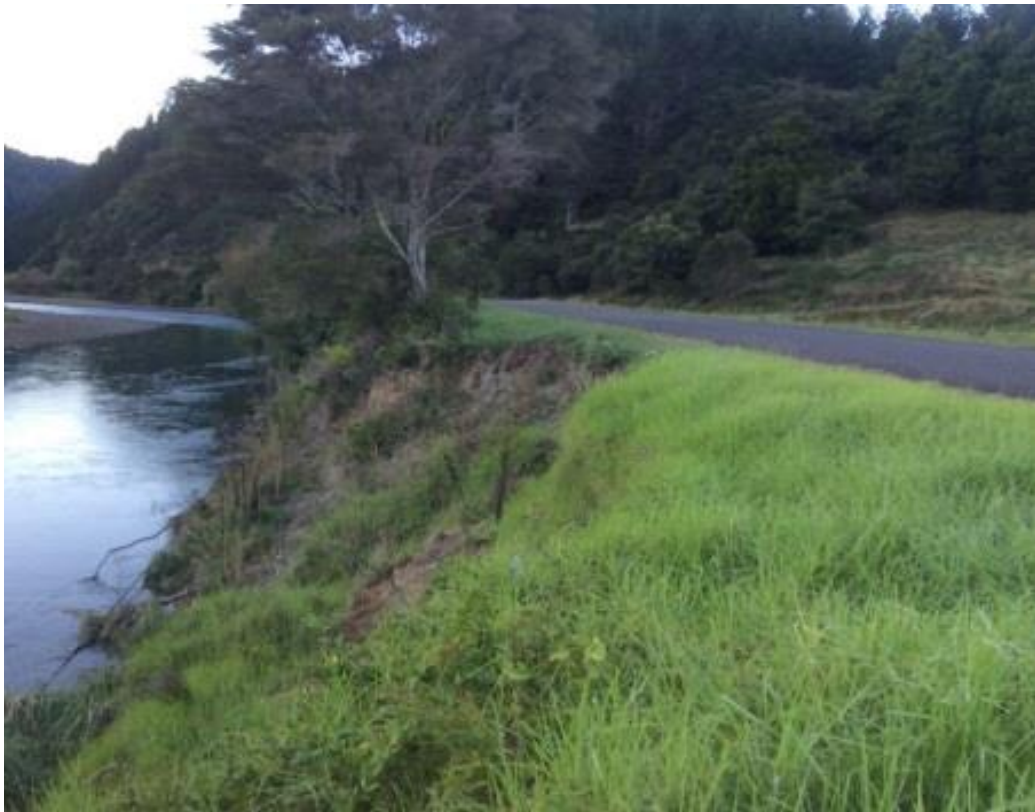
Photo 11: Pakihi Road no repairs as yet
