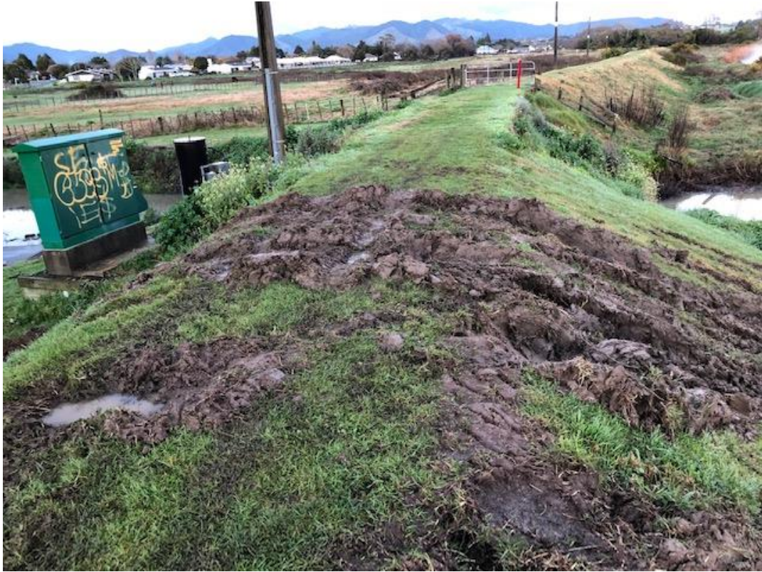
Photo 12: Stopbank damage at Tarawa Creek outlet
