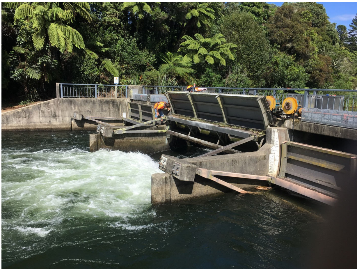
Figure 1 Okere Gates – Technicians calibrating the Okere Gates following replacement of the main lifting ropes – April 2019.
