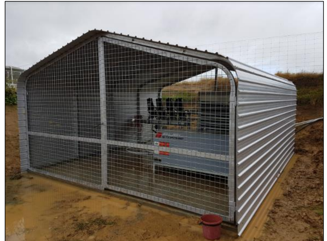
Proposed Presto Shed installation for both sites. With a solar panel or small transformer for lighting etc.
