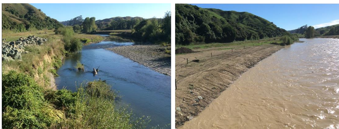
Figure 6: Waimana River at West Bridge - before (left) and after works completed (right). Note that in the right side photo the river is in flood and water levels are higher than the picture on the left.
