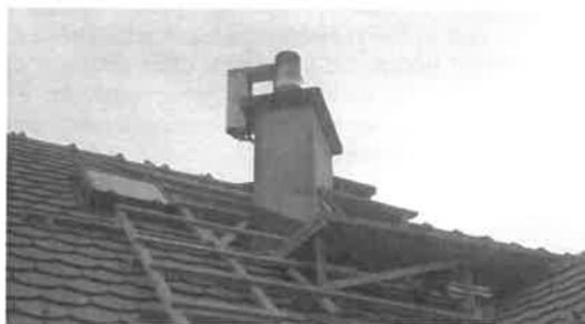
Figure 3: OekoTube mounted at site 2
