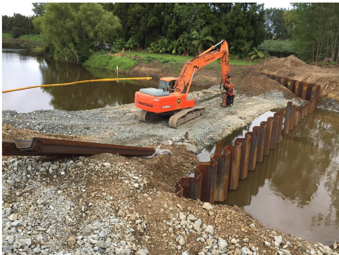
Figure 3. Kopeopeo Flood Control Structure – East under construction showing sheetpile installation with kink to avoid Whakatāne main sewer pipeline.
