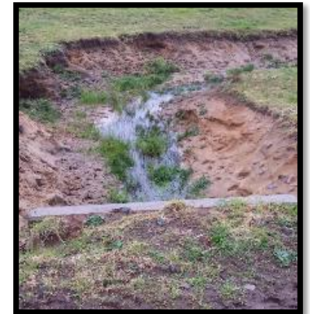
Figure 14 Stormwater Drain Discharging into Waipu Estuary 2013
