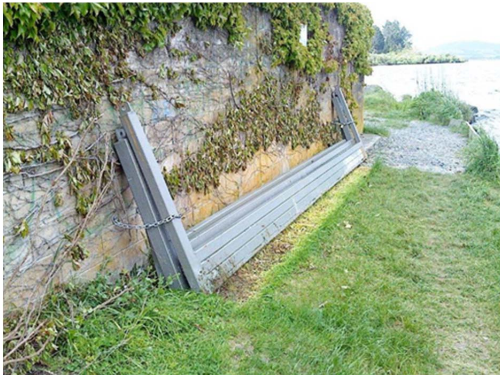
Figure 11 Ohau Channel stoplogs stored on site following refurbishment. Each stoplog is 6 m long x 0.3 m high.
