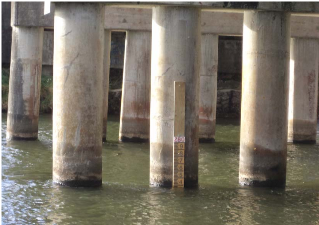
Figure 9 Ohau Channel/State Highway 33 staff gauge located on pillars of State Highway 33 Bridge at Mourea.
