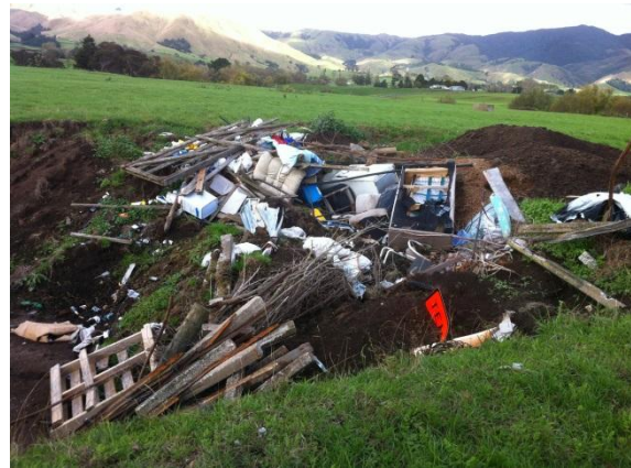
Figure 64 Deeper excavation on this farm dump means it can receive significant volumes of rural wastes
