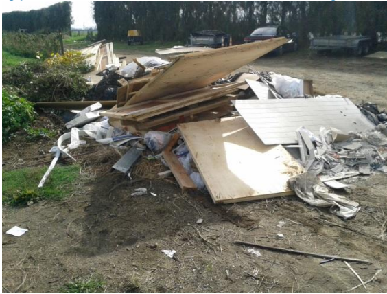
Figure 61 Demolition and mixed wastes about to be taken to farm dump and burnt
