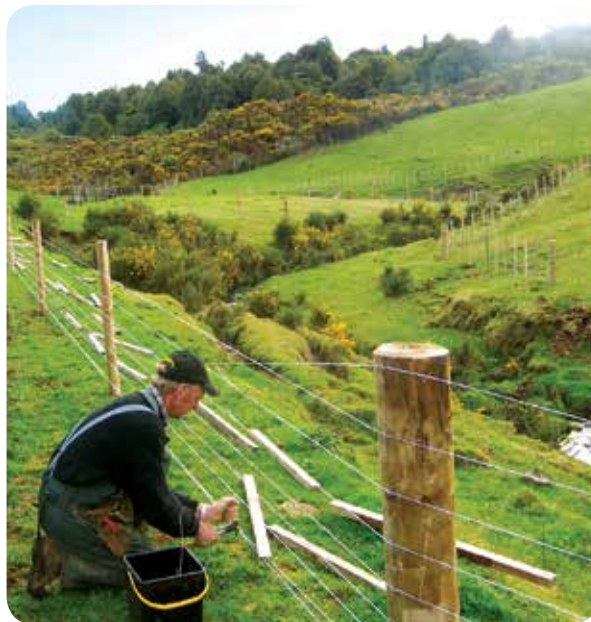
Photo: A fencing contractor constructs a 9-wire post and batten fence for riparian retirement.
