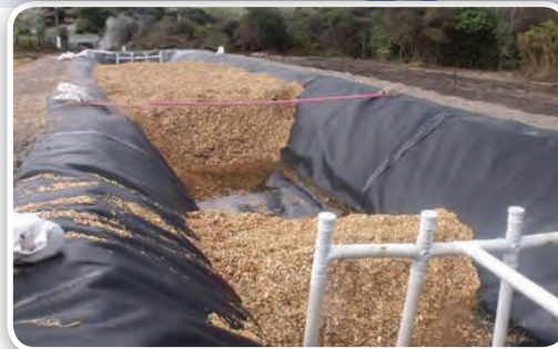
Tikitere pilot plant
